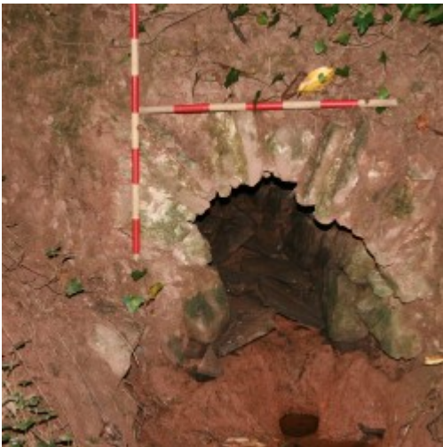
Buried deep in woodland, this drain outlet still carries water during heavy periods of rain
