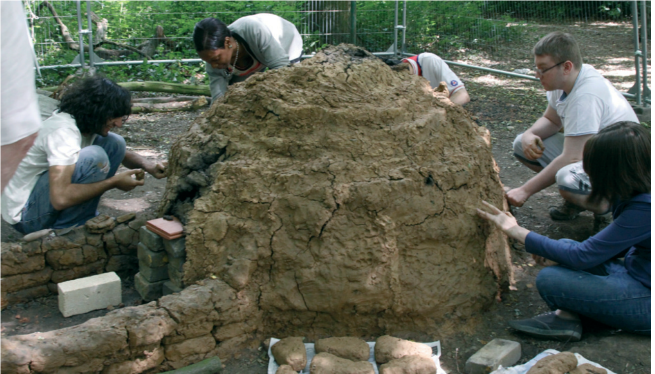
Fig. 5: Mathew, Nathalie, Omar, Tom and Jennifer repairing the fissures in the kiln. (Photograph: Bruce Castle Museum, Haringey Cultures, Libraries and Learning)
