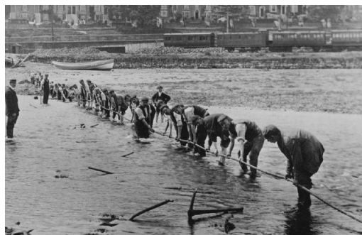
Fig 41 The laying of a cable in the River Esk © Sutcliffe Gallery ( www.sutcliffe-gallery.co.uk )
