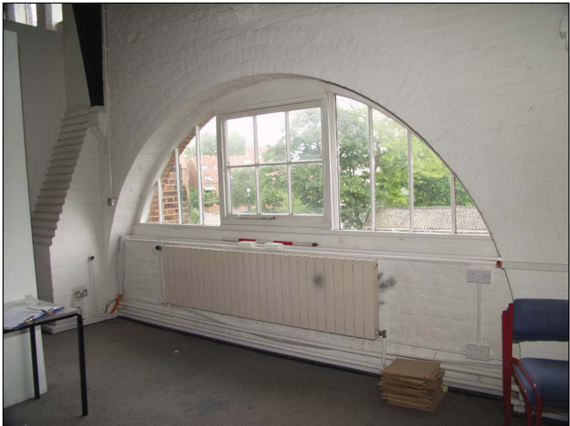
Plate 8 North-east wall of Bay 2 at upper level, taken from the south (DP 31)
