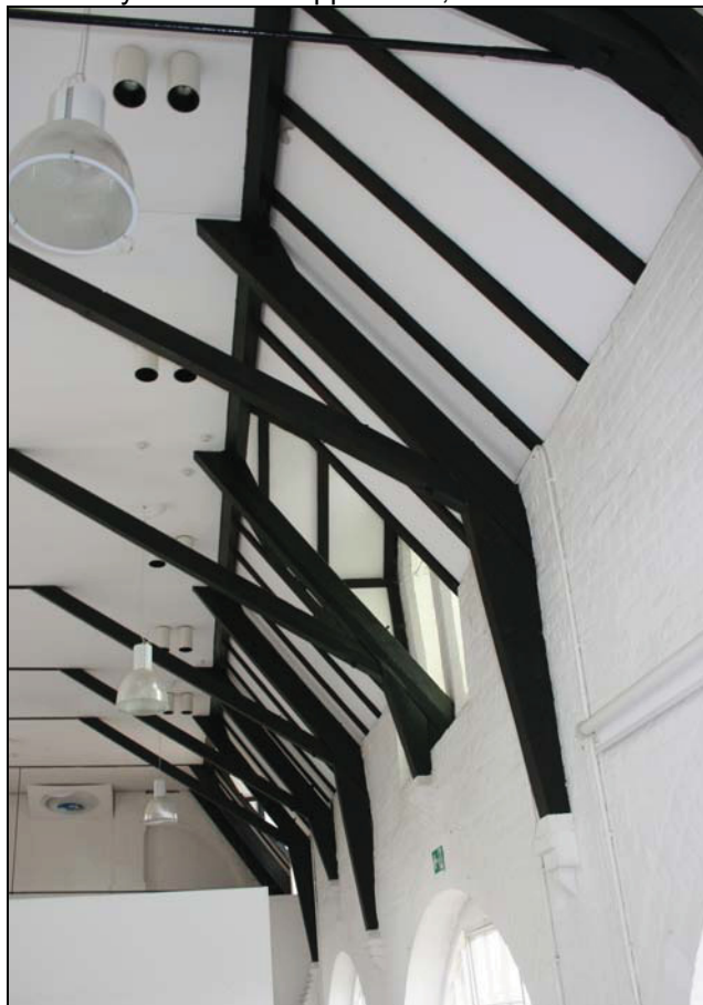
Plate 10 North-east side of the roof structure of the main building, taken from the south-east (DP 53)
