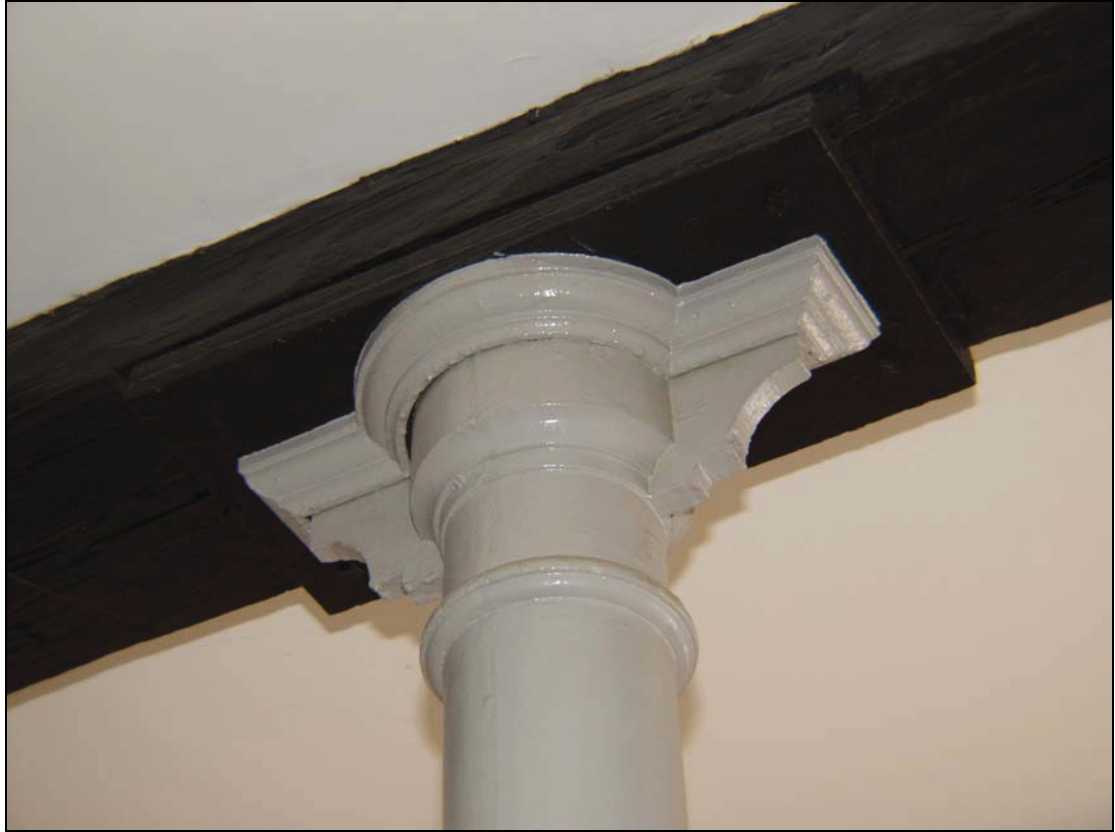
Plate 5 Detail of moulded head of the stanchions supporting the first floor, taken from the south-west (DP 21)
