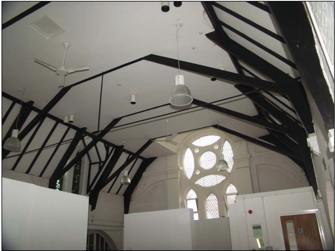
Plate 7 South-east area of the main building at first floor level, taken from the north-west (DP 37)
