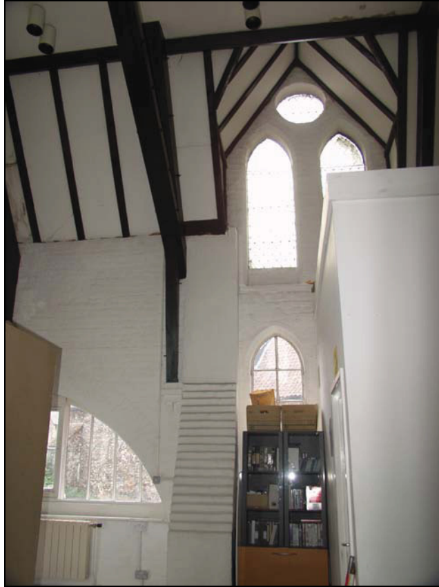
Plate 9 Division between Bays 2 and 1 at upper level, taken from the north-east (DP 32)
