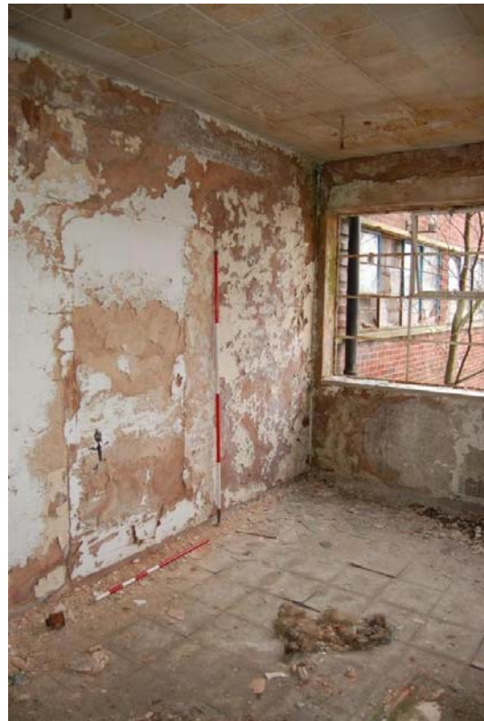
Plate 12: Bldg B1, 1 st Floor, blocked doorway to B2.
