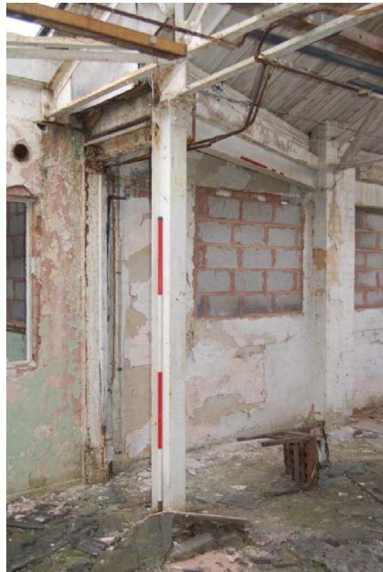
Plate 24: Bldg D 1st floor, angled trimmer (Bay 9) respecting location of former glass cone.
