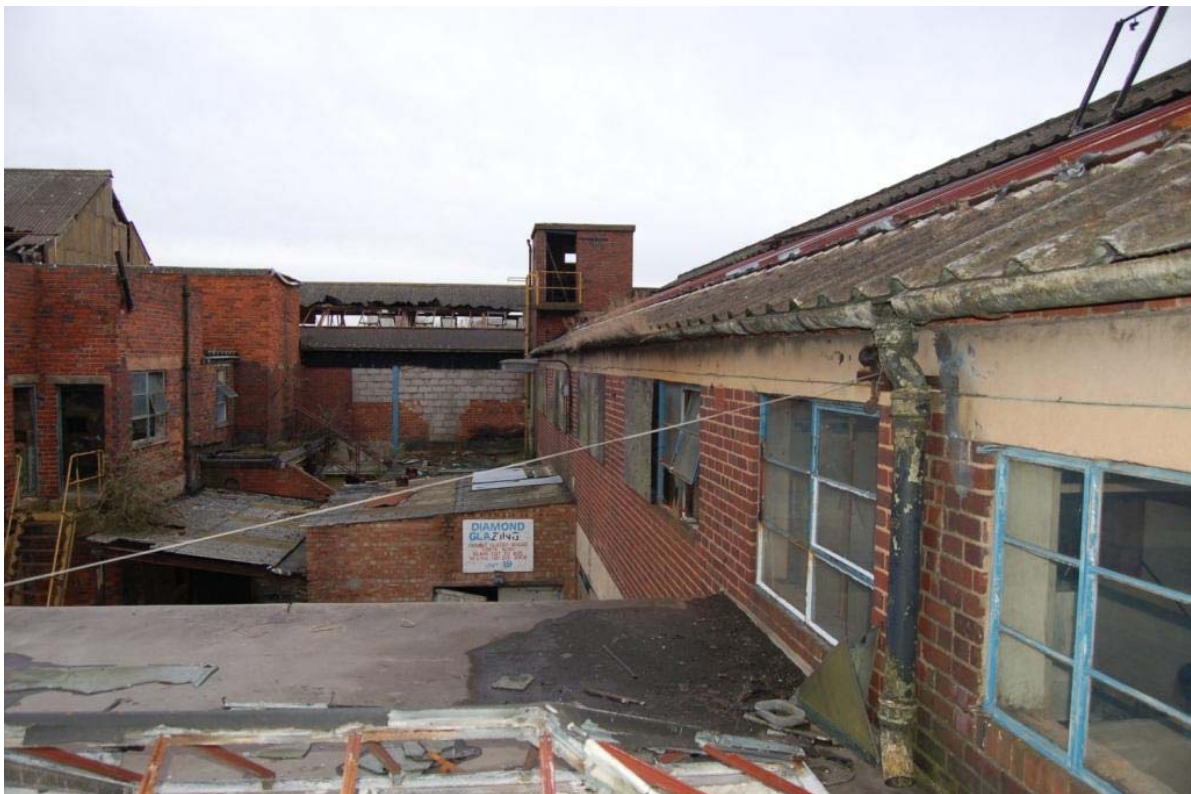
Plate 19: Building C, north elevation from roof of Building E, note lift shaft.
