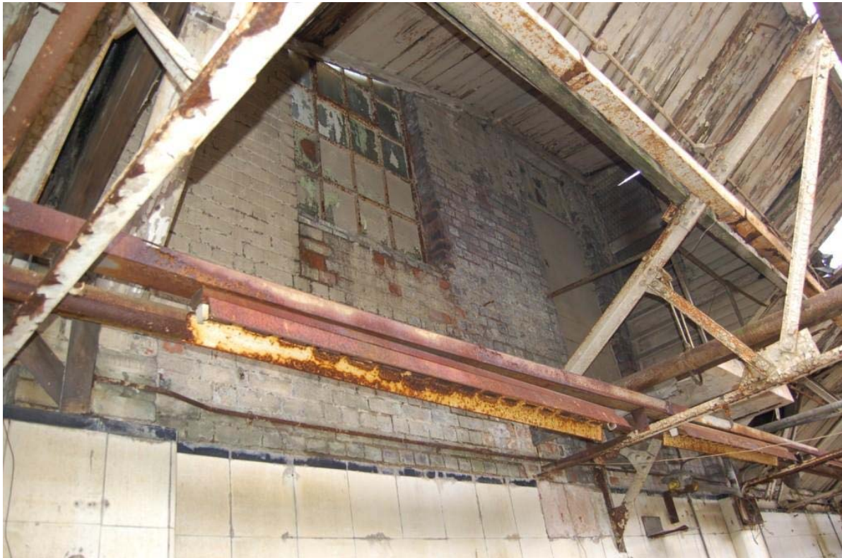
Plate 49: Building K, west wall; surviving early-c.20 th fabric including window (left) and door (right).
