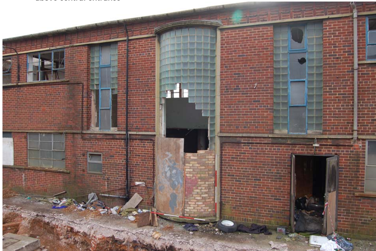
Plate 7: Building B1, rear elevation; detail of apsidal, glass block window lighting principal stair.
