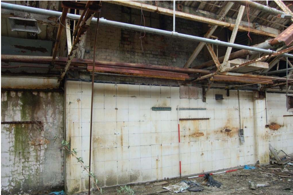
Plate 48: Building K, west wall; surviving early-c.20 th fabric, lined with white glazed tile at ground level.
