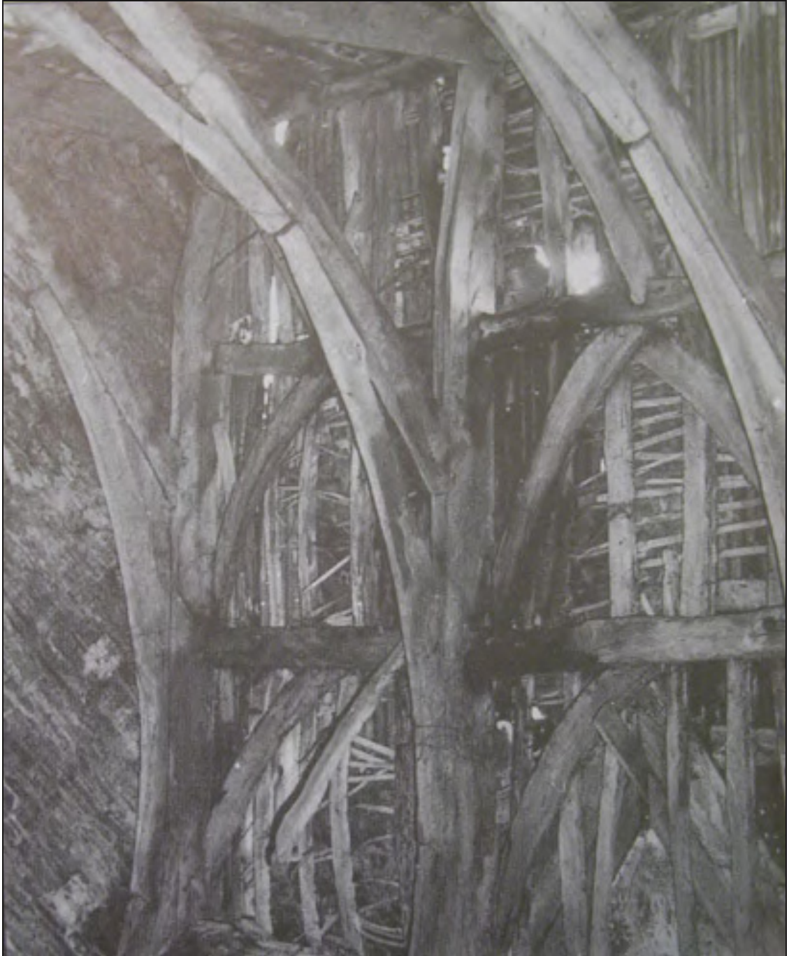
Figure 22: The original roof of the Great Barn, the western truss-blades at the southern end, viewed from below and to the north-east. This photo was published in Langdon (1995), and shows the 15 th century arch-braced roof was in a poor state of repair by the early-mid 20 th century.
