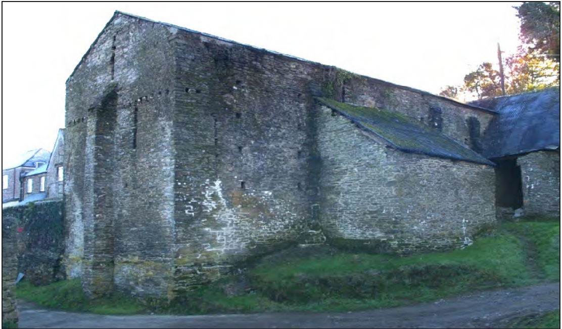
Figure 17: North and west elevations of the Great Barn, viewed from the north-west.
