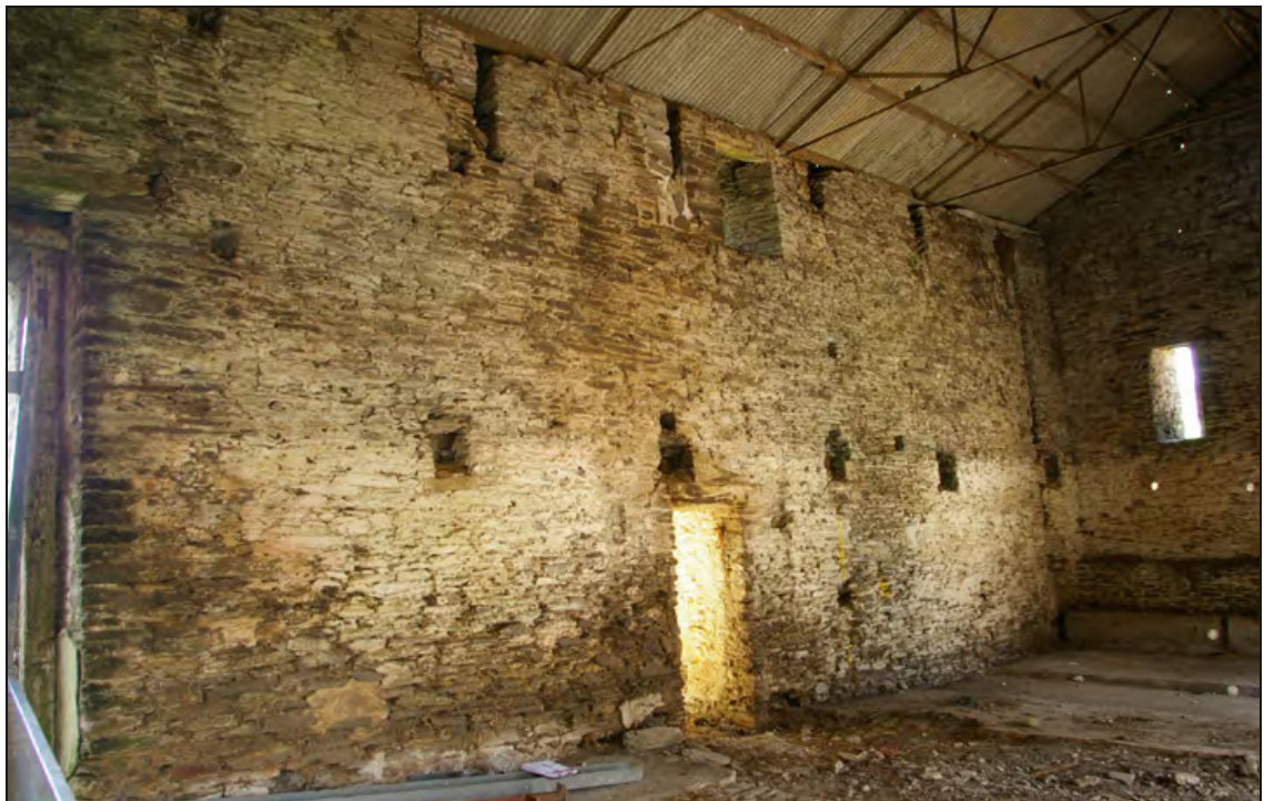
Figure 21: The interior of the Great Barn, the north end of the west wall, viewed from the south-east.
