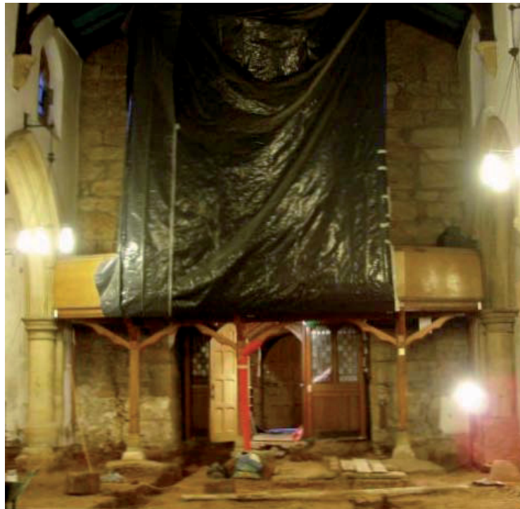
Plate 13: The roof scars visible on the east side of the tower (west end of the nave), either side of the tarpaulin
