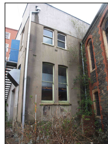
4.9 View of the north west corner of the church hall abutting the church
