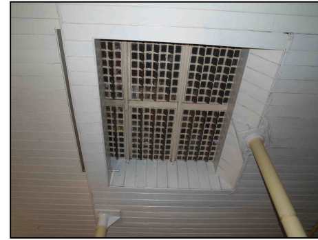
6.3 View of underside of ceiling light in Room G1.
