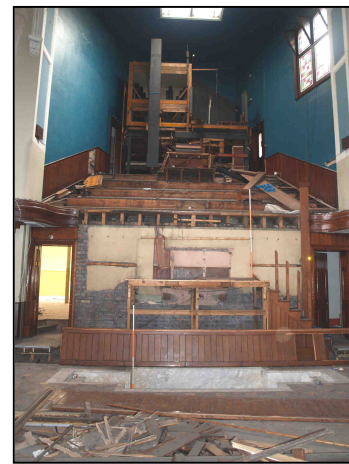
4.2 View of partially dismantled organ, pulpit framework and Baptismal Pool at east end of church.
