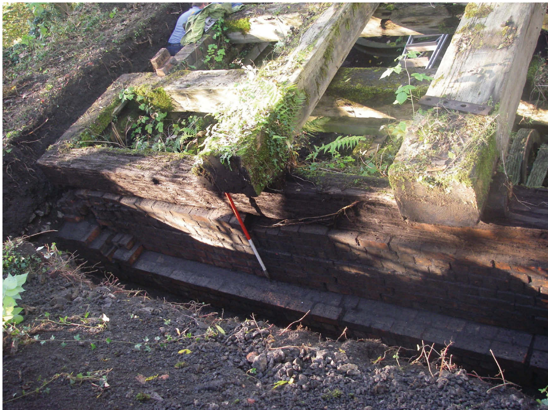
Plate 5: Eastern end of pit, looking south-west. Note cracking and subsidence at south-east corner (left of photo).
