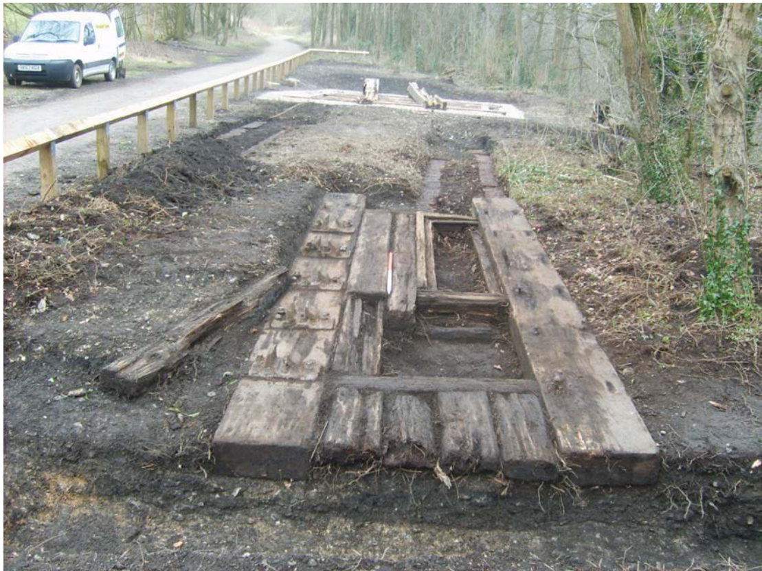
Plate 2: General view of timber structure [304], with both cable runnels behind, leading to the wheel pit. Looking east
