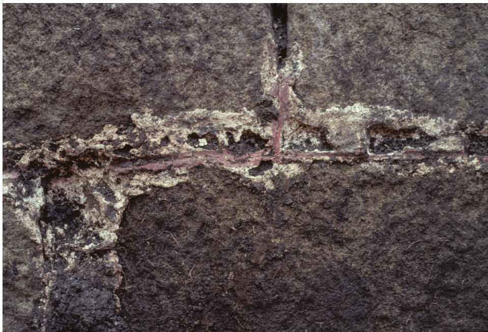
Fig. 16: Site A. the north face of the corner turret showing the 'false jointing'. The detail below shows how the grooves were picked out in red paint.
