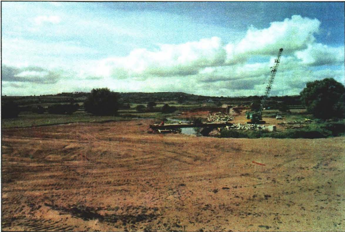
Pl. 4 Construction work in Yarty flood plain, the River Yarty is in the foreground. Looking west
