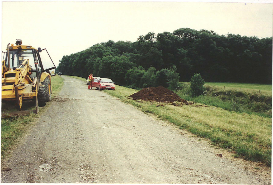
Pl. 1 Position of Trial Trench A on the west side of the track. The Car Dyke is to the west of the trench, with Nocton Wood beyond. Looking south.
