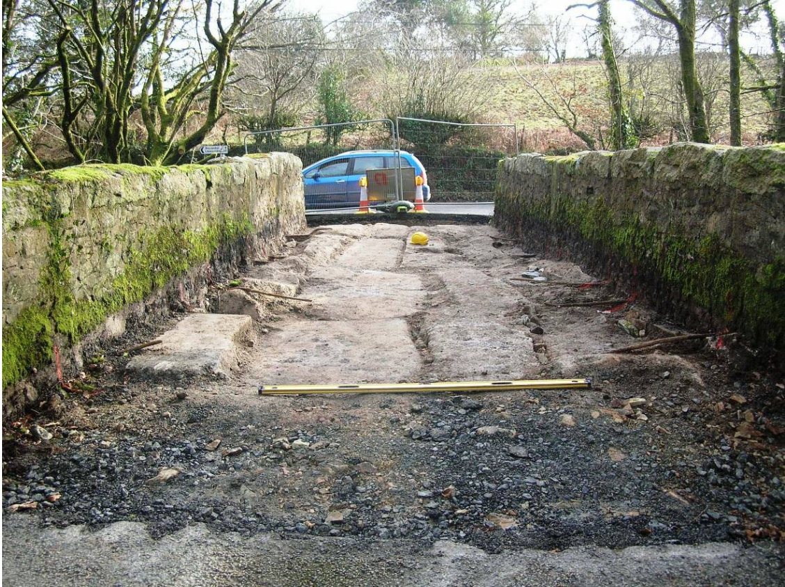
Fig 21 Draynes Bridge after removal of the road surface, January 2013 (looking E) The spirit level used as a scale is 6ft (1.83m) long
