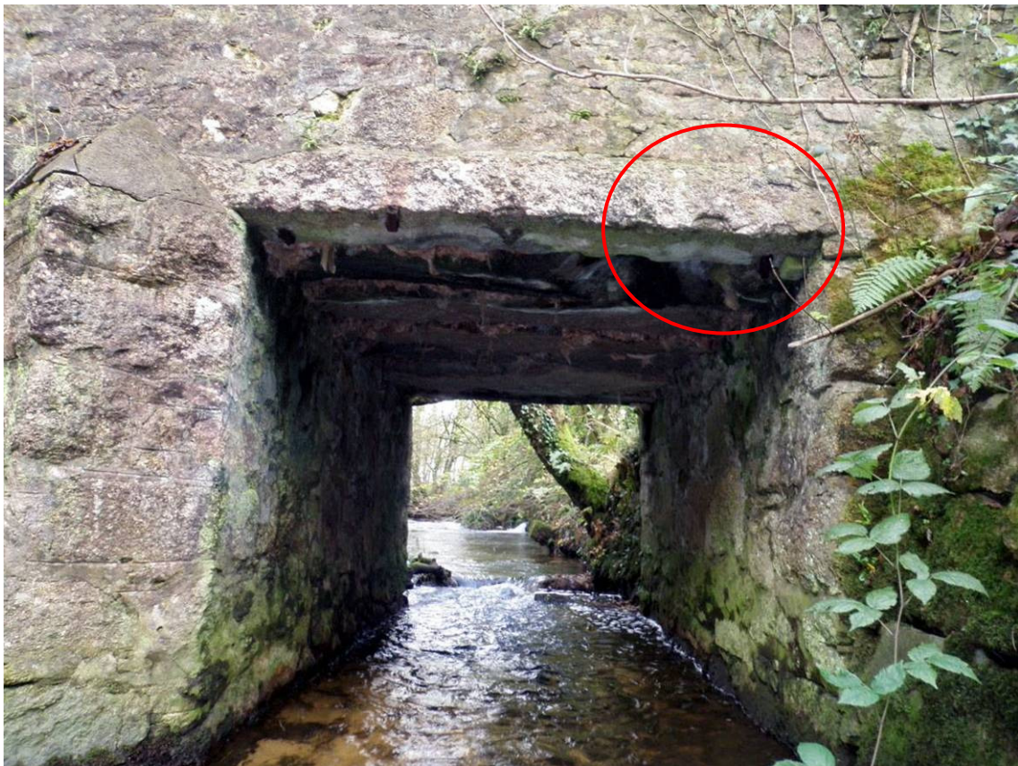
Fig 18 The eastern span of the bridge has evidence of pre-1800s wedge splitting
