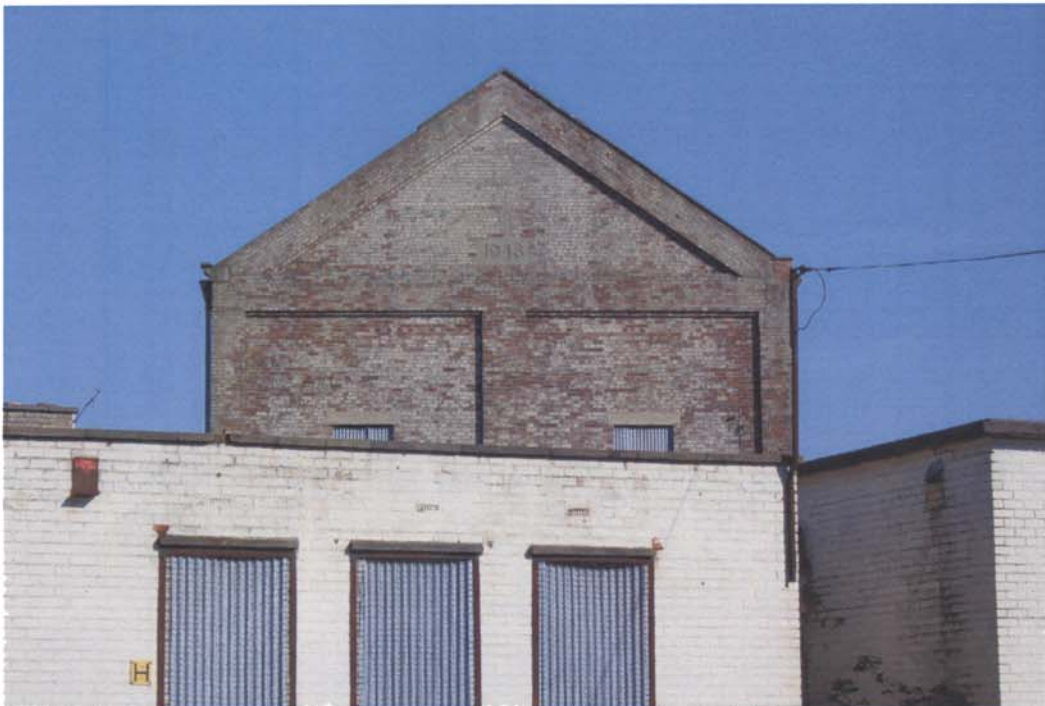
Plate 24. Former winding house, dated 1946, to the west of the study site, looking east.
