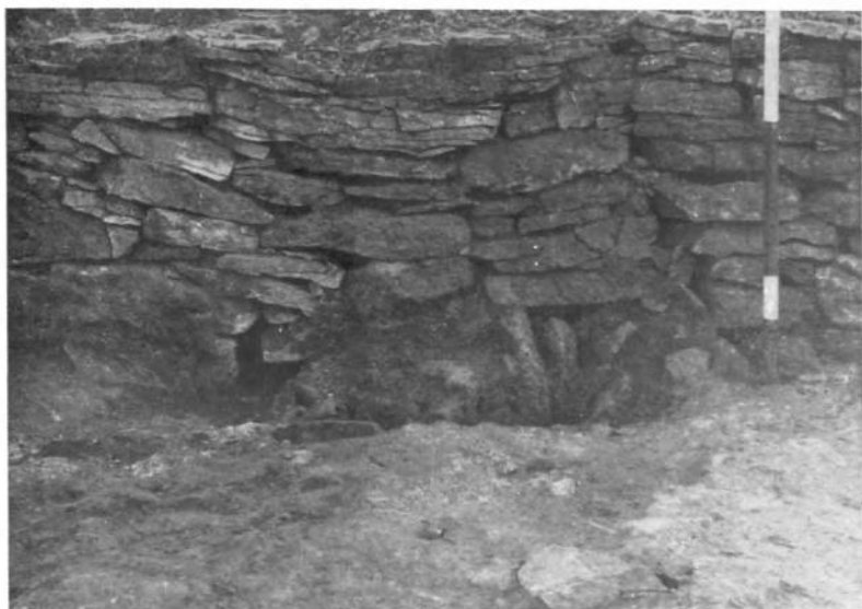
A. SUBSIDENCE OF THE S. WALL OF THE NW. SIDE-ENTRANCE INTO THE FILLED IN POST-HOLE OF A PREVIOUS GATE. NOTE THE STRAIGHT JOINT WHERE ADDITIONAL WALLING WAS ADDED
