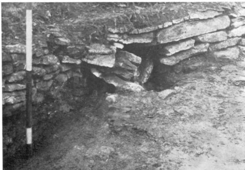
B. JOINT AT SUBSIDENCE OF THE N. WALL. NOTE HERE ALSO THE ROUGHER STONES USED FOR THE LATER WALLING
