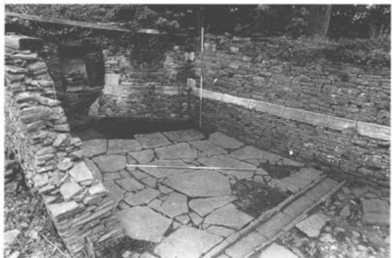
Figure 4.26 The standing south wall of the west range from the south-east (photograph: Robert Bell).
