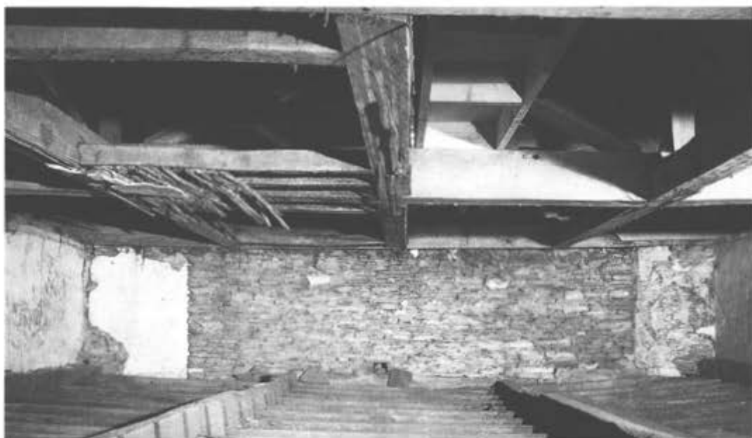
Figure 5.16 East range: above the lowered ceiling, showing the blocked north window, Period 4.1 frieze and remnants of the original ceiling (photograph: English Heritage B870019/11).
