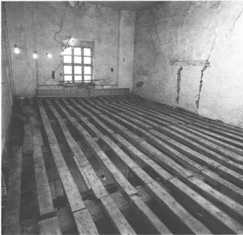
Figure 4.6 Room 11 looking south showing the floor joist structure (photograph: English Heritage B870005/1).
