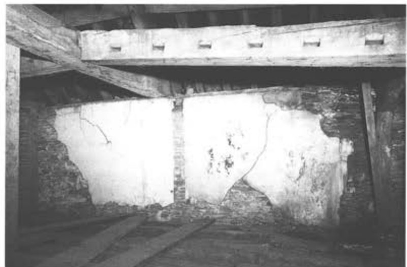
Figure 4.8 Period 4.1 partition scar in the east range roof space (west wall) (photograph: English Heritage B870019/14).
