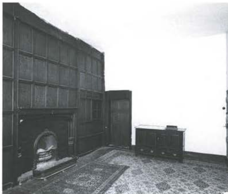
Figure 7.4 Room 6: the lowered ceiling is set at the base of the Period 4.1 frieze and the Period 4 panelling is reset (photograph: © Crown copyright. NMR BB98/00609).
