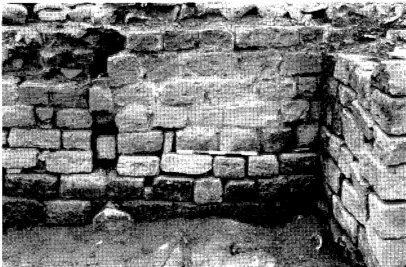
Fig 81 Surviving pointing on outside of south wall of Building 197 (18)
