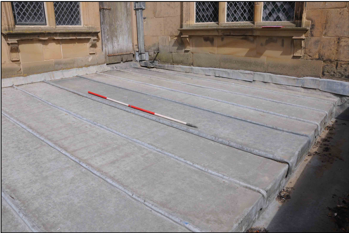
Appendix I.10: Detail of lead roof sheets in Section A, looking north-west (2m scale) (Photo D20)
