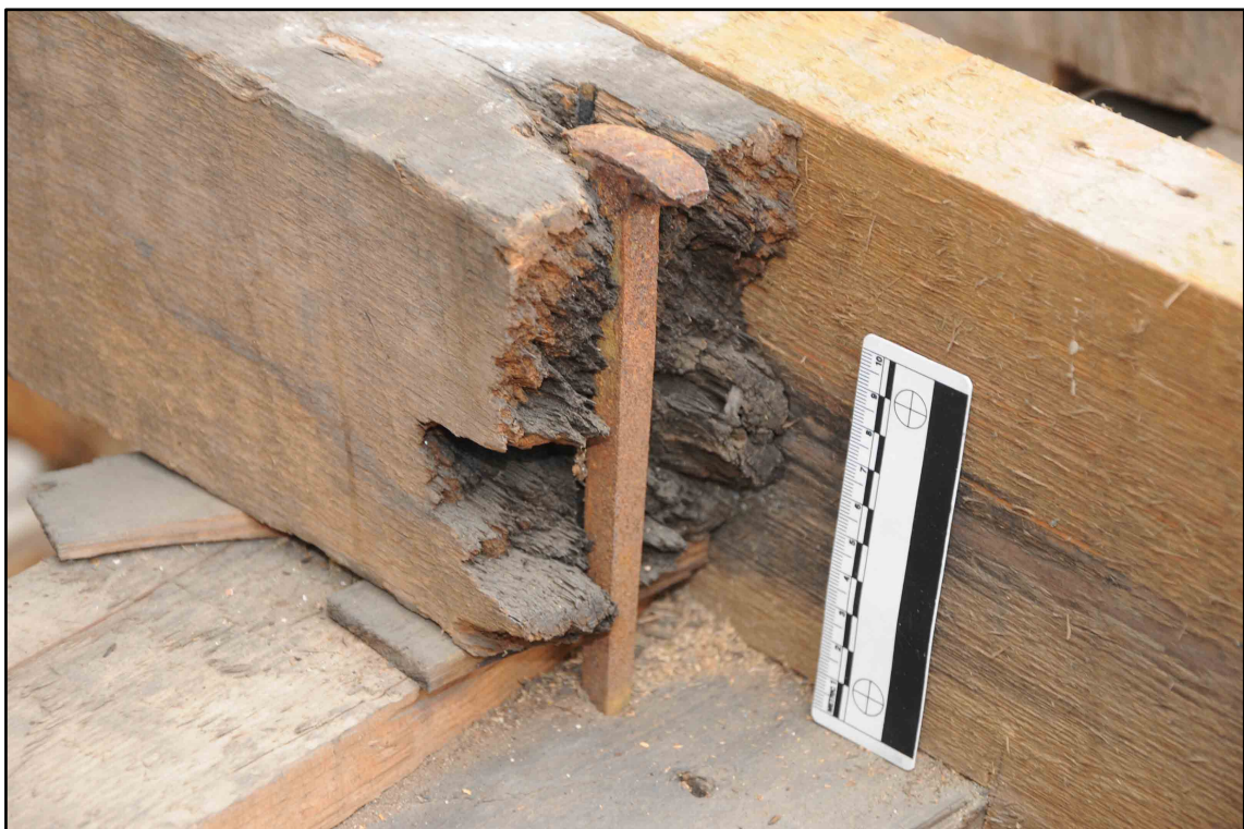
Appendix I.31: Detail of purlin in Section E; note assembly iron peg (10cm scale) (Photo D174)
