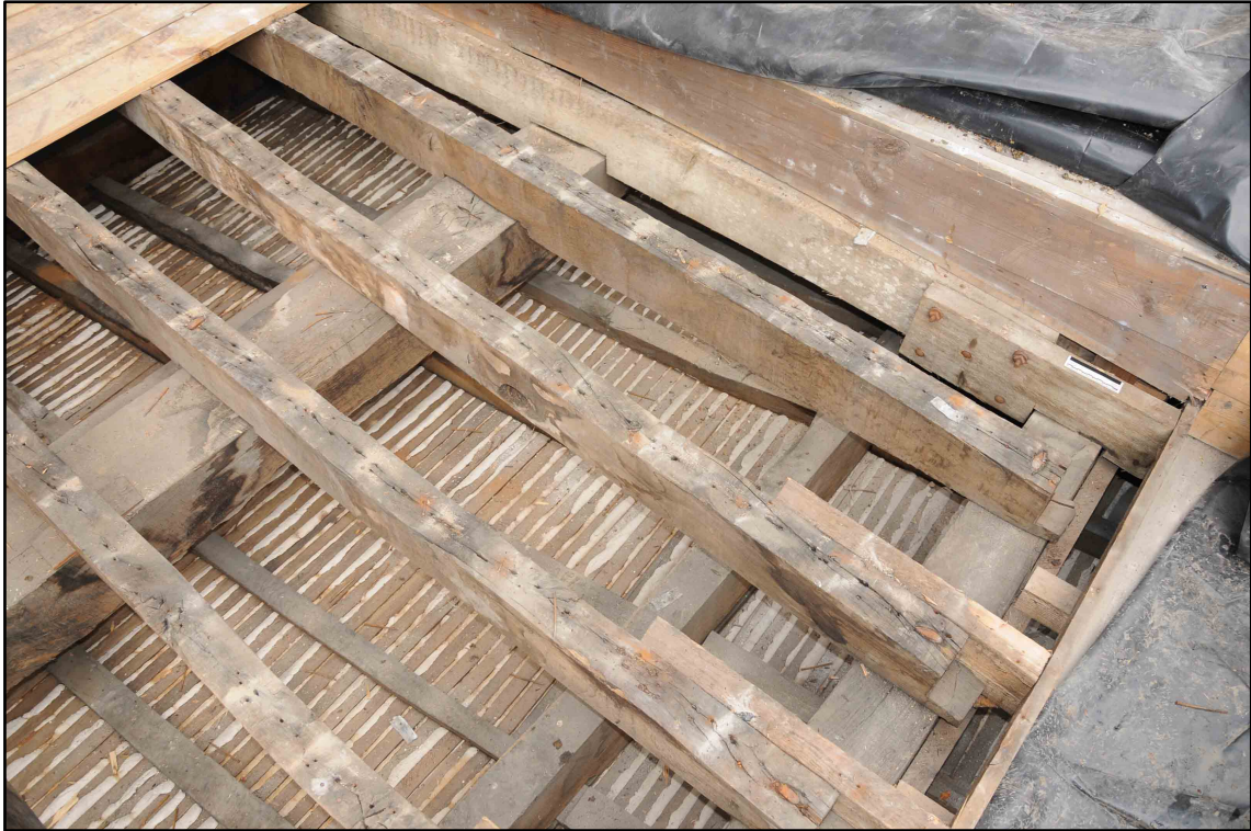
Appendix I.28: Detail of roof structure in Section E/D, looking north-west (10cm scale) (Photo D168)
