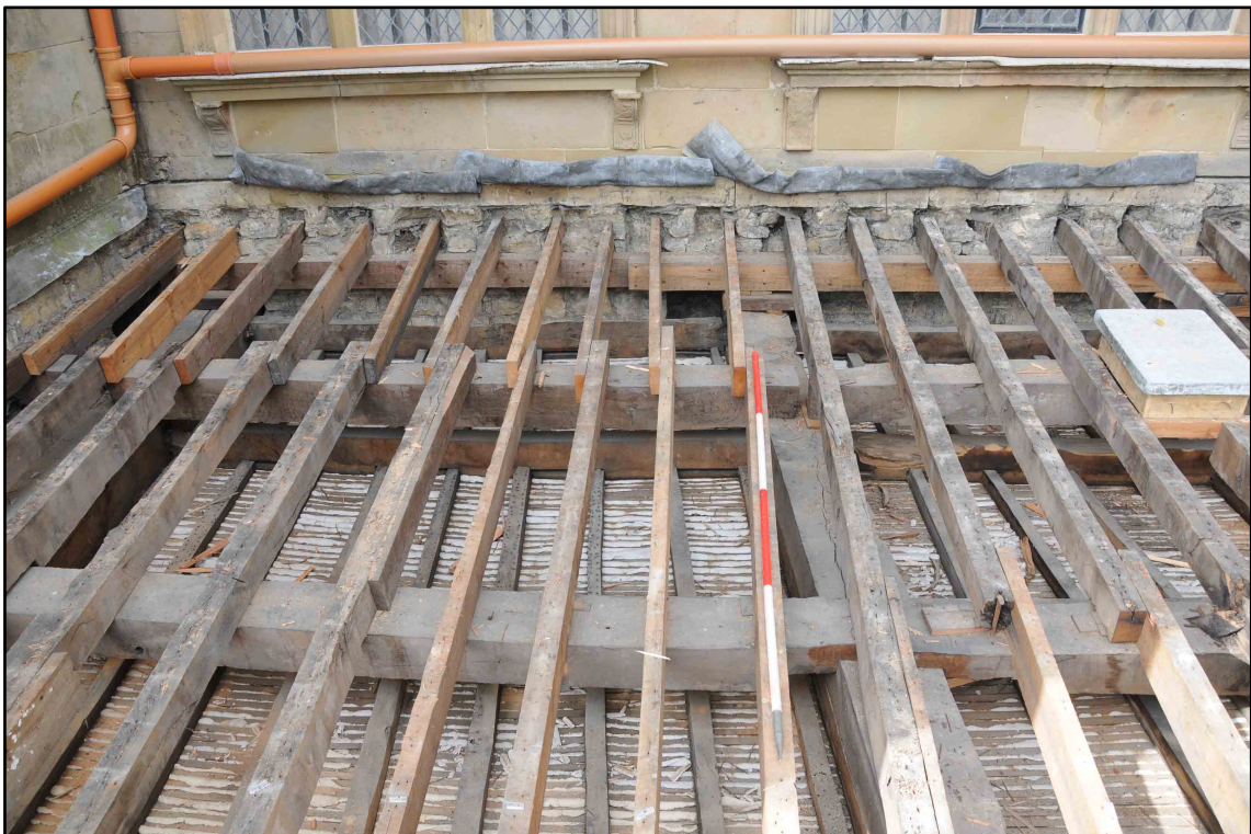
Appendix I.29: Detail of roof structure in Section E, looking west (2m scale) (Photo D178)
