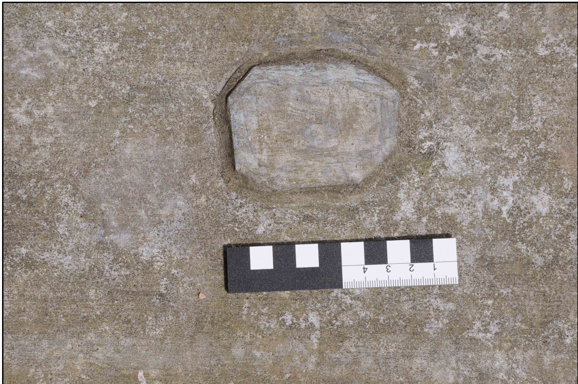
Appendix I.20: Detail of lead patch repair in Section C (10cm scale) (Photo D64)
