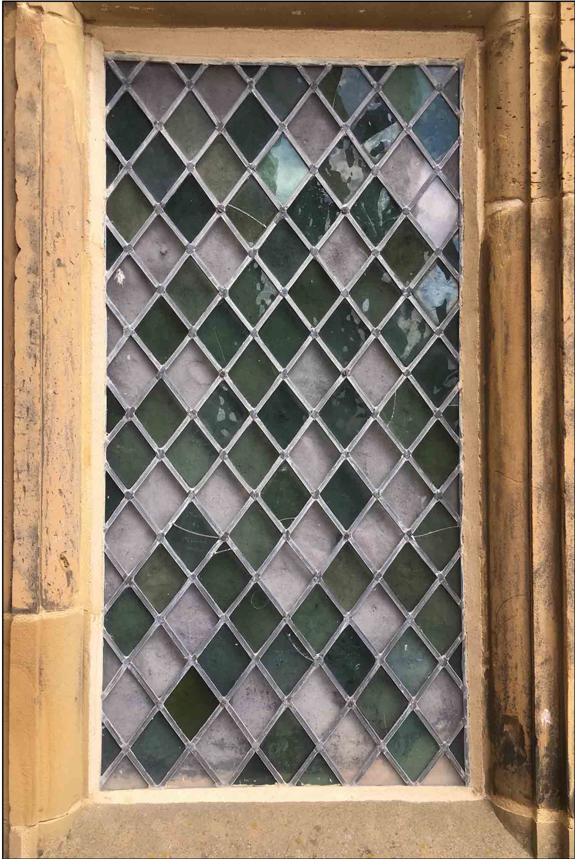
Appendix I.50: Detail of (false) north window (W126) with graffiti (Photo D11)
