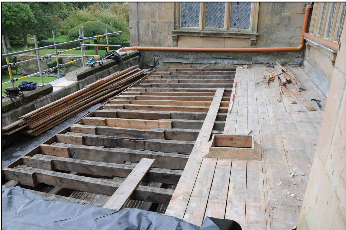
Appendix I.13: View looking south across Section E during removal of boards (2m scale) (Photo D115)
