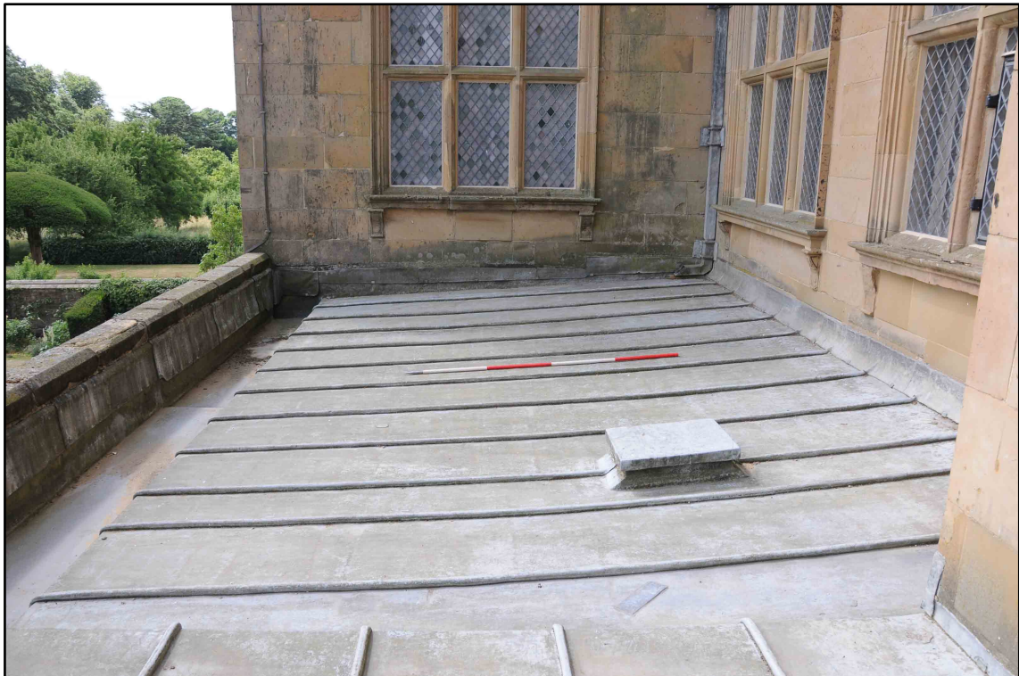
Appendix I.12: View looking south across Section E prior to works commencing (2m scale) (Photo D49)
