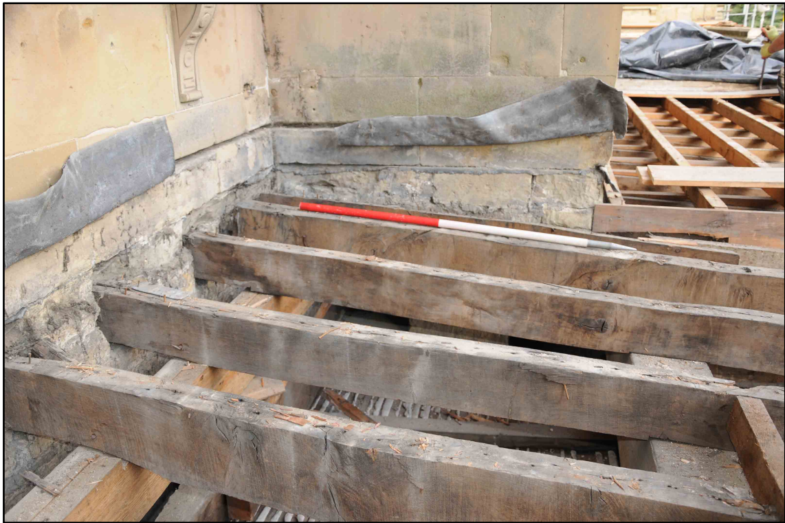
Appendix I.40: Detail of primary oak rafters in north-west corner of Section E (1m scale) (Photo 194)
