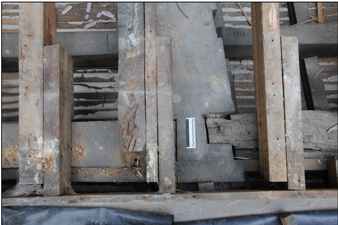
Appendix I.27: Detail of roof structure in Section E, looking east (10cm scale) (Photo D142)
