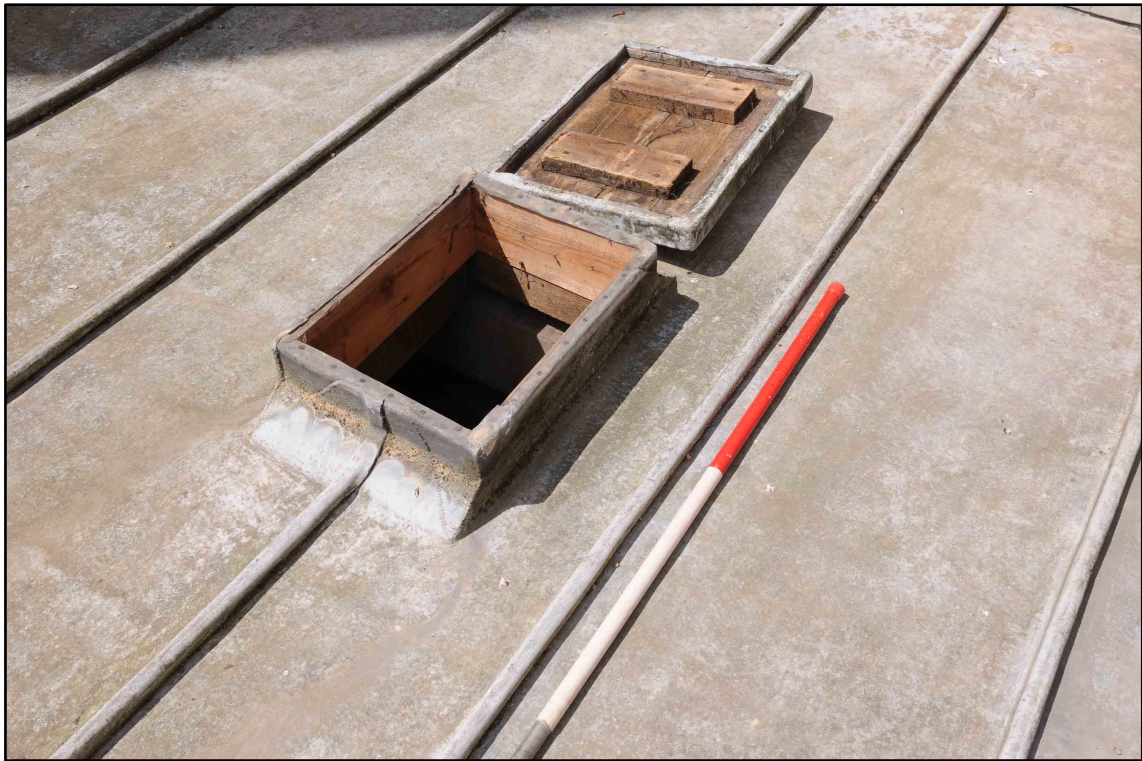
Appendix I.18: Detail of hatch in Section E, looking south-west (1m scale) (Photo D70)
