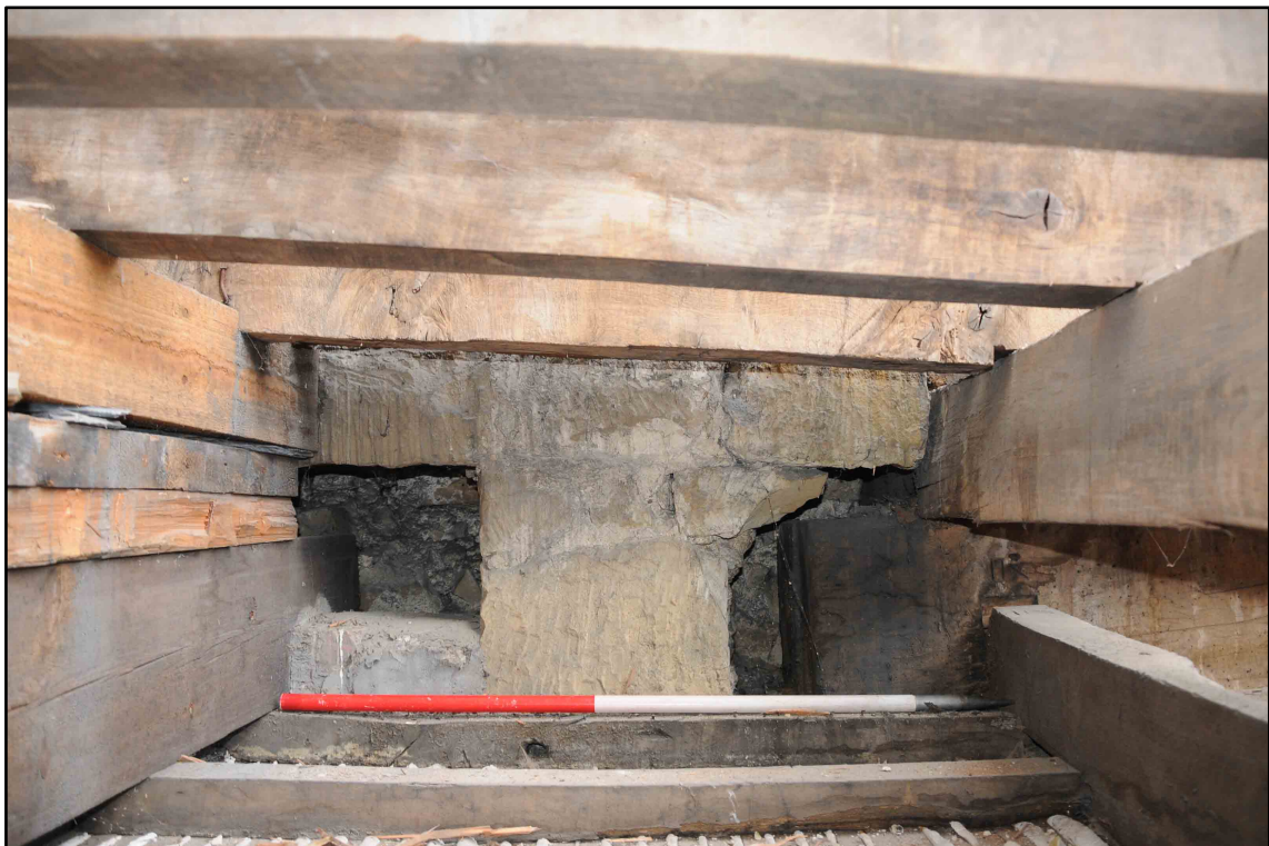
Appendix I.41: Detail of sockets within masonry of central bay of the east facade (1m scale) (Photo DI97)
