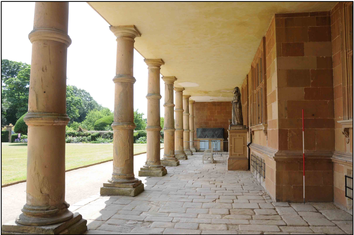
Appendix I.3: Detail of collonade below East Loggia, looking south (2m scale) (Photo D94)
