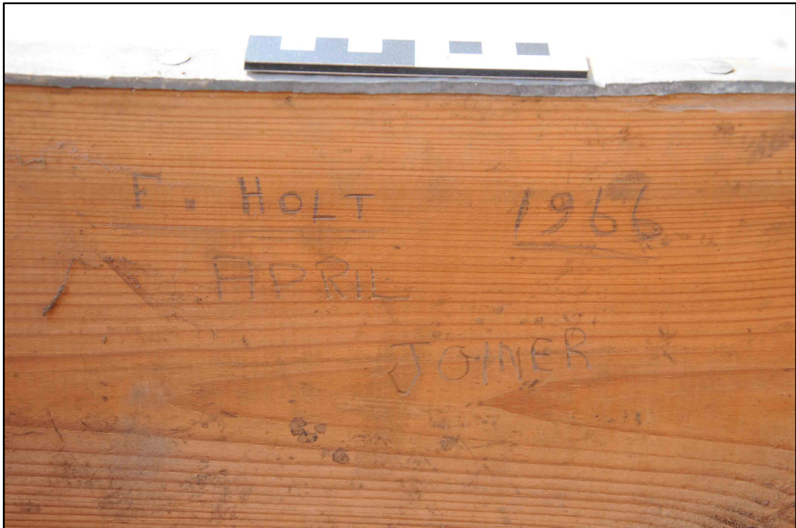
Appendix I.16: Graffiti in hatch in Section A 'F.Holt April Joiner 1966' (10cm scale) (Photo D27)
