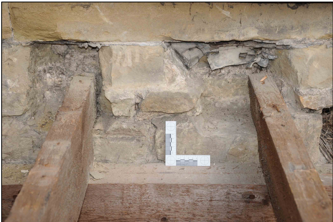
Appendix I.39: Detail of cut sockets for secondary rafters in Section E (5cm scale) (Photo D192)
