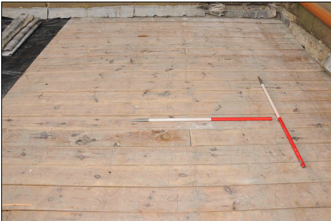
Appendix I.11: Detail of pine boards below leads in Section A, looking west (1m scale) (Photo D169)
