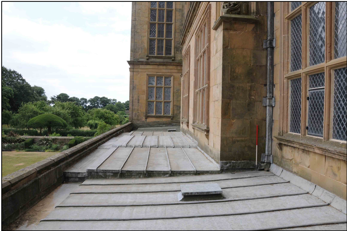
Appendix I.7: General view looking south of East Loggia roof before restoration (1m scale) (Photo D77)
