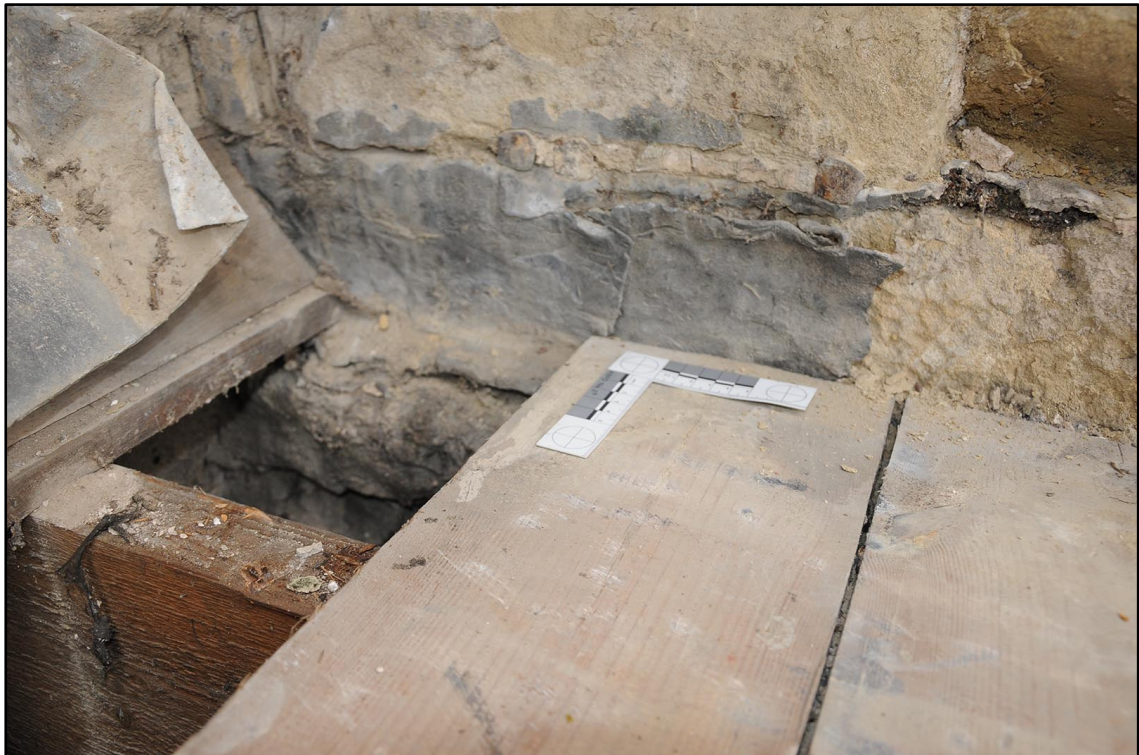
Appendix I.47: Detail of original lead flashing bent down below pine boards (5cm scale) (Photo D171)
