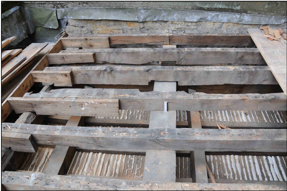
Appendix I.26: Detail of roof structure in Section E, looking south (10cm scale) (Photo D145)
