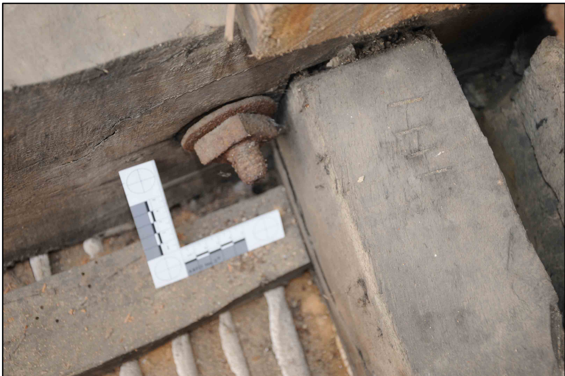
Appendix I.33: Detail of iron bolt (repair?) in south-west corner of Section E (5cm scale) (Photo D186)
