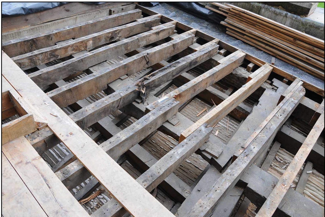
Appendix I.25: Detail of roof structure in Section E, looking north-east (Photo D148)
