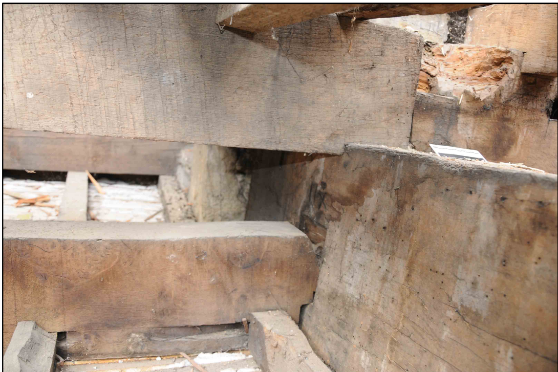
Appendix I.45: Detail of roof timbers at junction of Sections D and E (10cm scale) (Photo D204)
