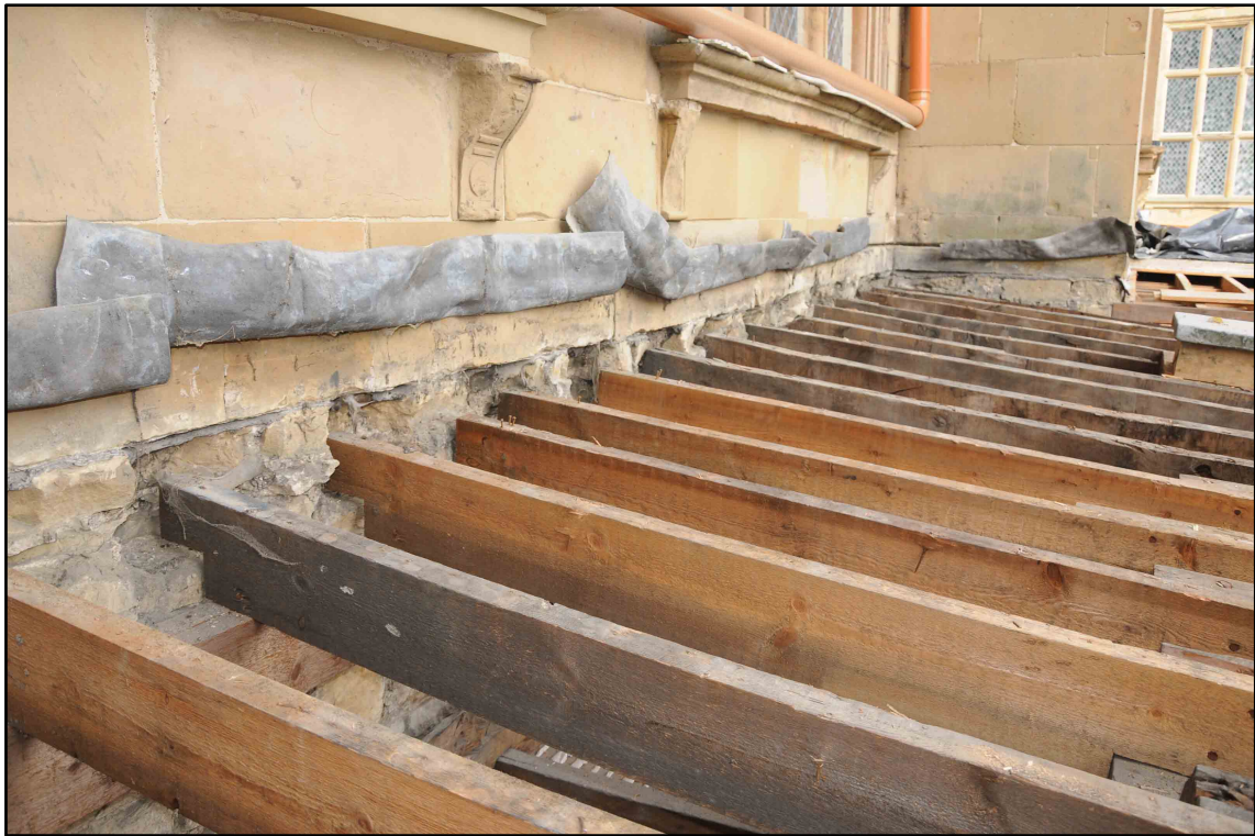
Appendix I.38: View looking north-west along replaced rafters in Section E (Photo D193)
