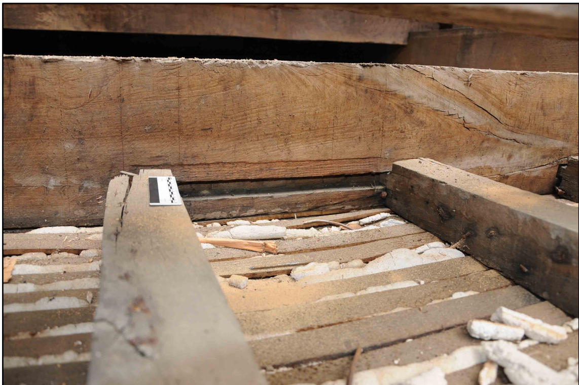
Appendix I.35: Detail of tenon and groove for lower joists in Section E (10cm scale) (Photo D156)
