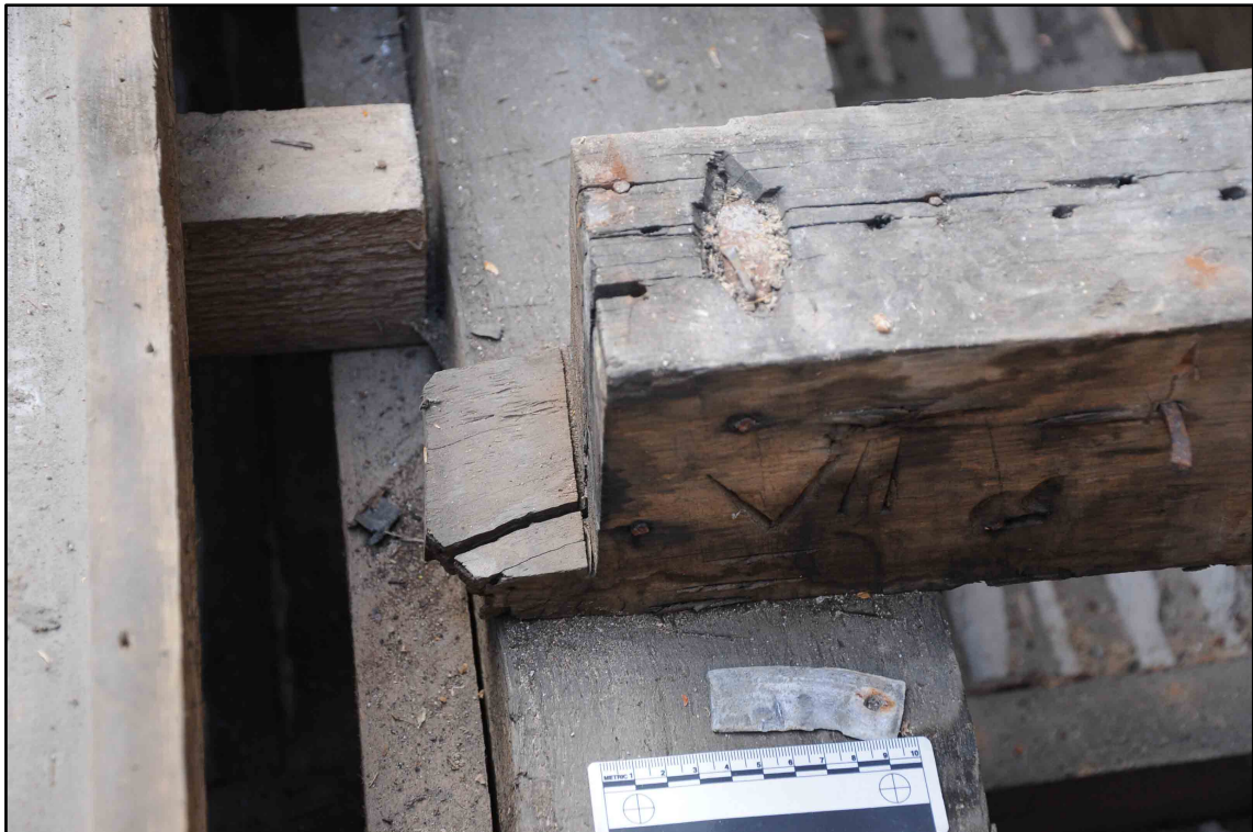
Appendix I.30: Detail of purlin in Section E; note assembly mark and iron peg (10cm scale) (Photo D205)
