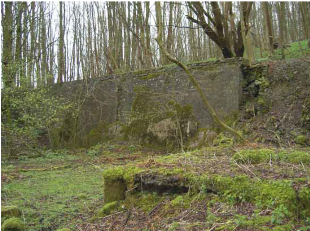
Figure 56: Blast wall BW4 behind the mark II large corning house, looking north-east (Photograph: Christopher Dunn 2006, © English Heritage)
