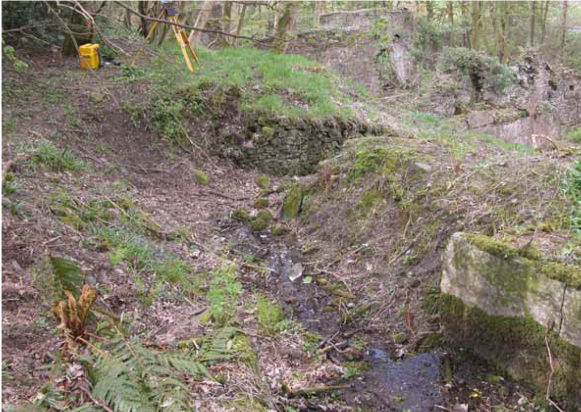
Figure 10: The south end of the mill leat and start of the sloping culvert (Photograph: Christopher Dunn 2006, © English Heritage)
