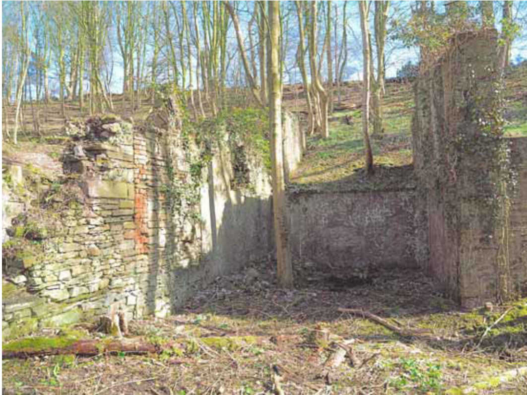
Figure 40: The south chamber of incorporating mill 5, showing later extension westward (Photograph: Bob Skingle 2006, DP028071 © English Heritage.NMR)
