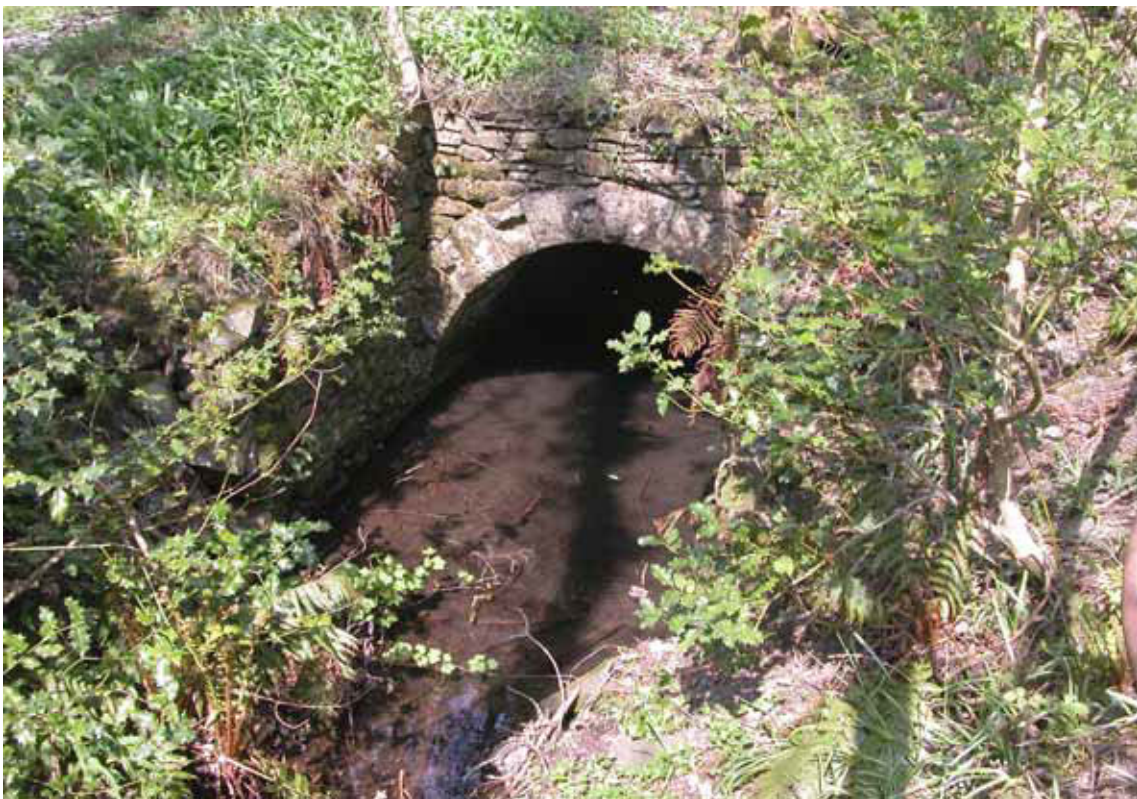
Figure 13: The exit portal of the low-level culverted leat north of Challon Hall (Photograph: Christopher Dunn 2006, © English Heritage)
