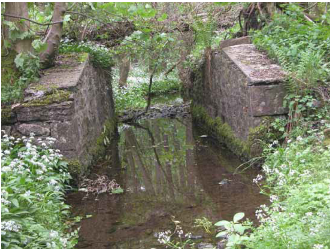
Figure 103: Bridge abutments on the tram spur to the press houses (Photograph: Christopher Dunn 2006, © English Heritage)
