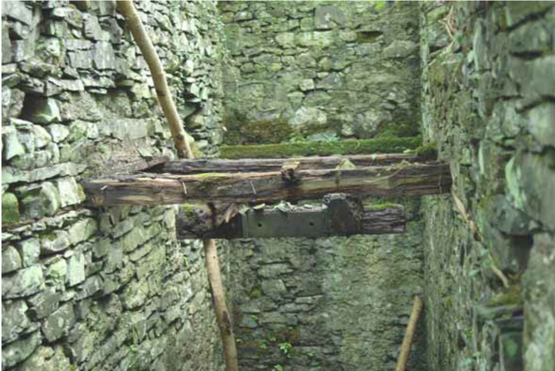
Figure 34. Timber framework supporting the drive shaft from the turbine in incorporating mill 3 (Photograph: Christopher Dunn 2008, © English Heritage)
