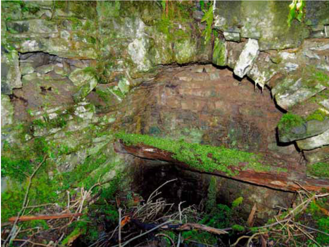
Figure 32: Blind arch in waterwheel house in incorporating mill 7 (Photograph: Bob Skingle 2006, DP028081 © English Heritage.NMR)
