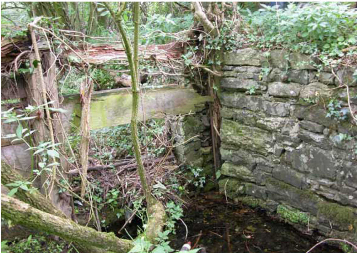
Figure 9: The sluiceway at the head of the gunpowder mill leat (Photograph: Christopher Dunn 2006, © English Heritage)
