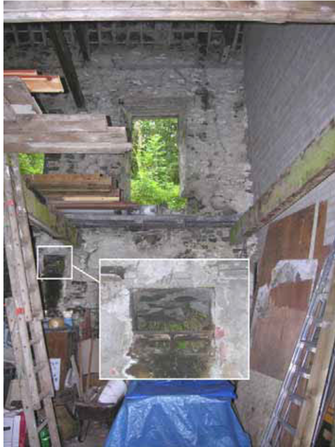
Figure 87: Interior view of the rear wall of the sawmill/mechanics' shop, with bearing box shown in detail at inset (Photograph: Simon Taylor 2006, © English Heritage)
