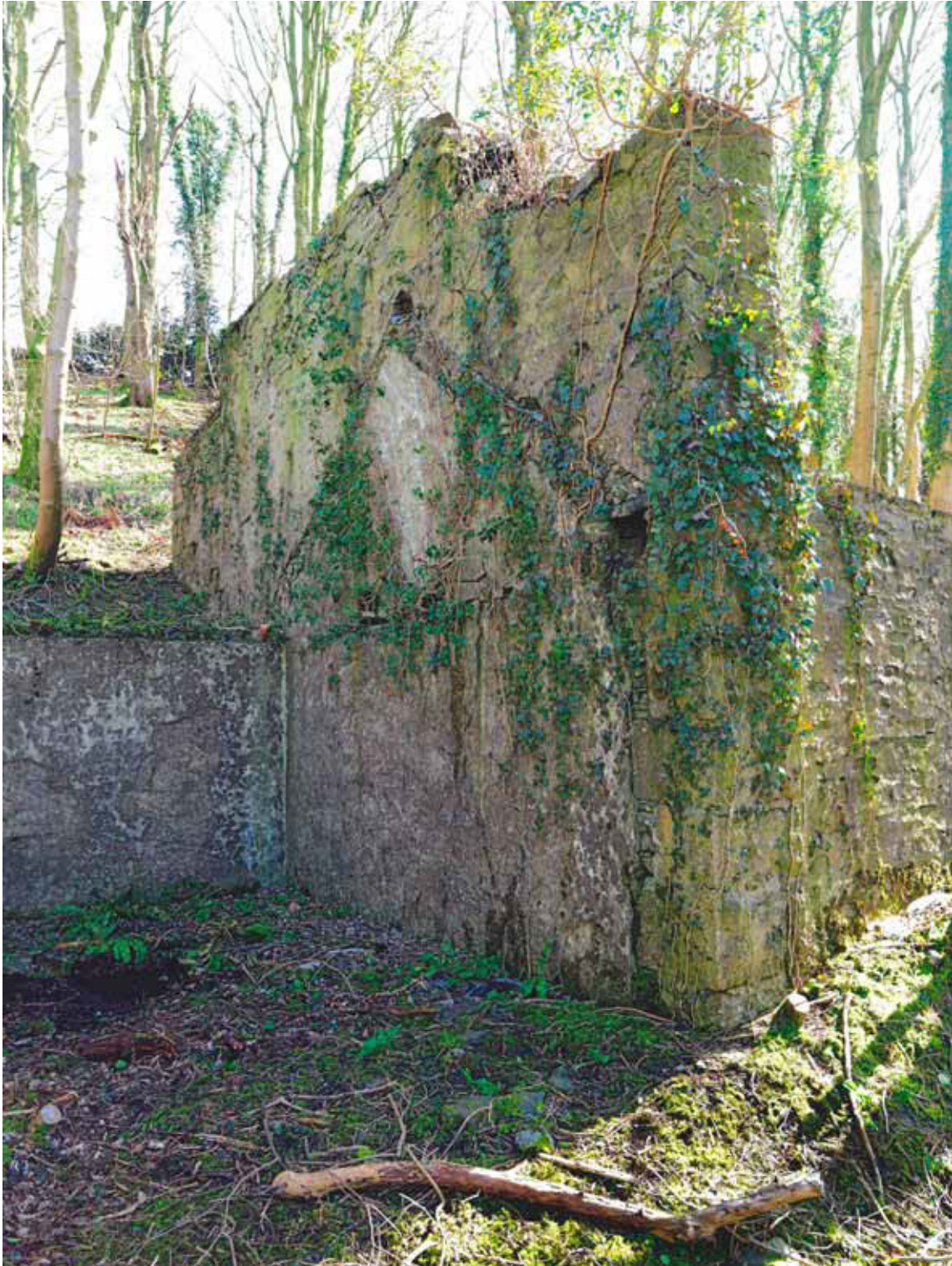
Figure 25: The south wall of the south chamber of incorporating mill 5 (Photograph: Bob Skingle 2006, DP028072 © English Heritage.NMR)
