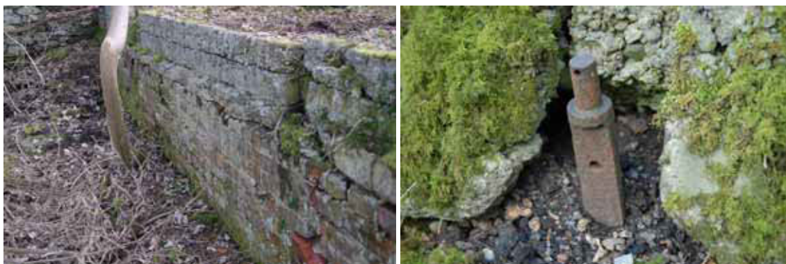
Fig 94 (above left): Detail of the north-east end of the floor slab of the infill building
