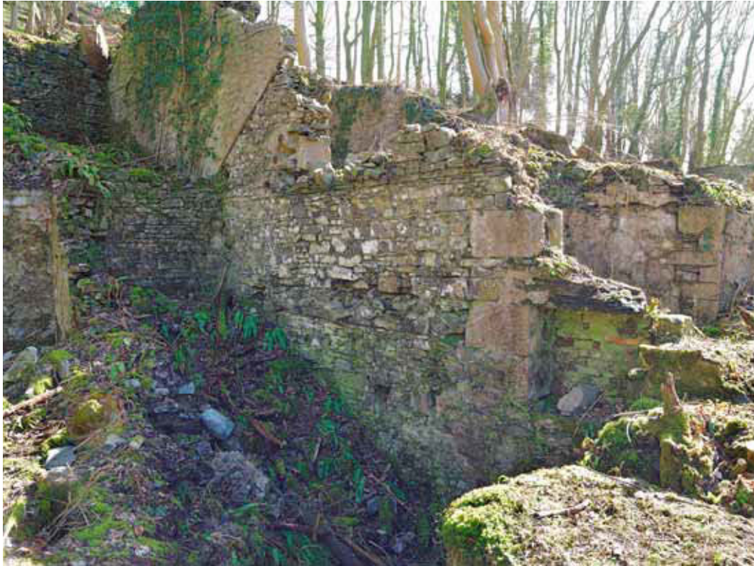
Figure 28: The waterwheel house and drive-shaft aperture at incorporating mill 7 (Photograph: Bob Skingle 2006, DP028080 © English Heritage.NMR)
