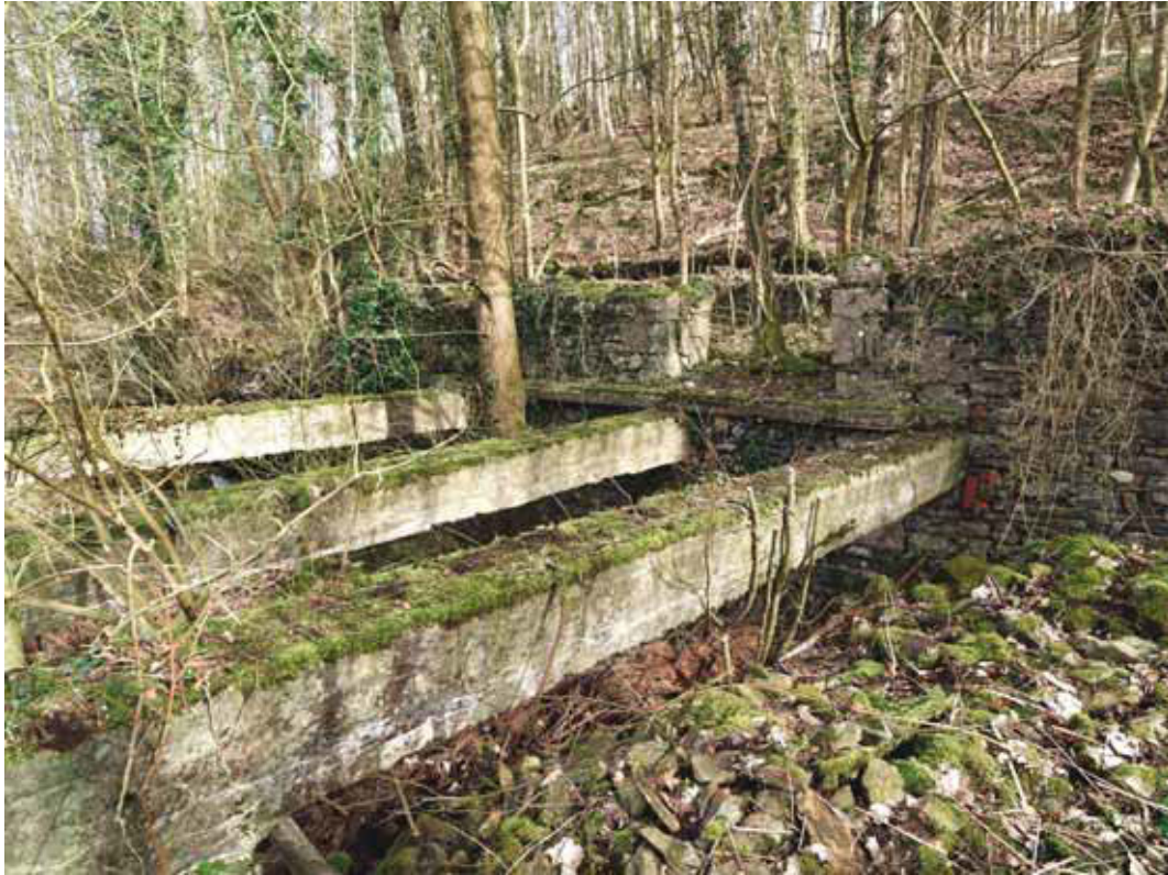
Figure 92: Joists spanning the mill leat at the joiners' shop (Photograph: Bob Skingle 2006, DP028090 © English Heritage.NMR)
