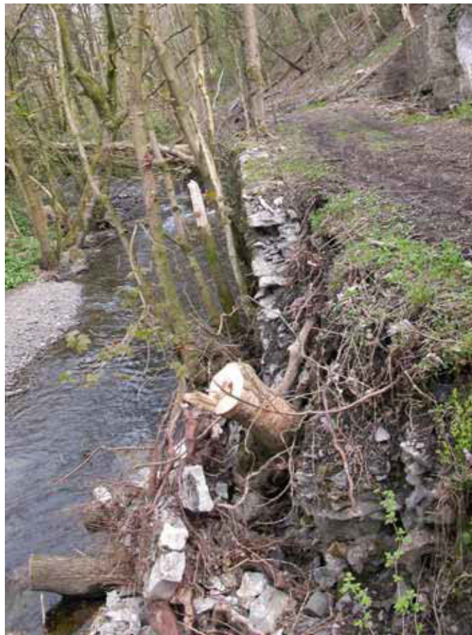
Figure 3: Collapsed stream revetment opposite the northern charge house (building 6) (Photograph: Christopher Dunn 2006, © English Heritage)
