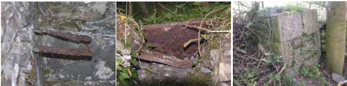
Figure 80 (above left): Iron pins in the rear wall of the watch house Figure 81: (above middle): inspection cover at top of wall flue Figure 82 (above right): The watch-house chimney (building 4a) (All photographs: Christopher Dunn 2006, © English Heritage)
