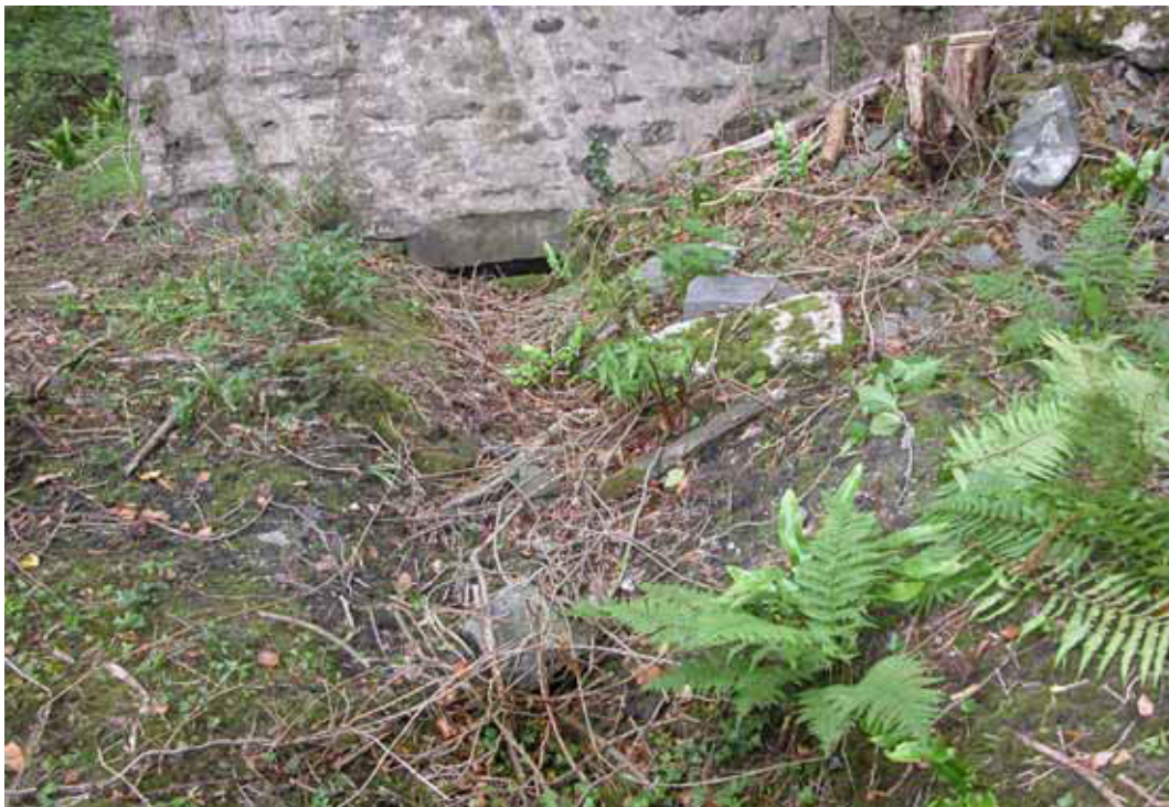
Figure 37: Detail of the wall of incorporating mill 3 extended over the turbine race (Photograph: Christopher Dunn 2006, © English Heritage)
