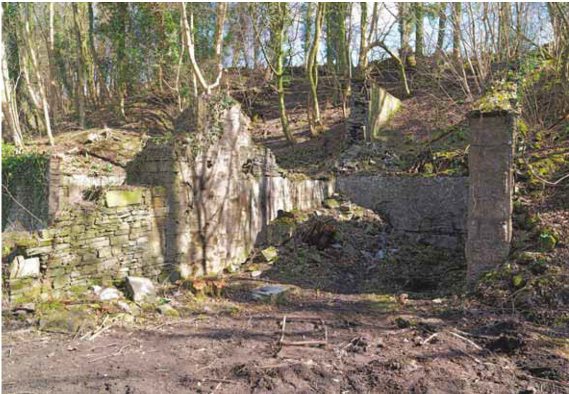
Figure 19: The south chamber of incorporating mill I following tree clearance (Photograph: Bob Skingle 2006, DP028056 © English Heritage.NMR)
