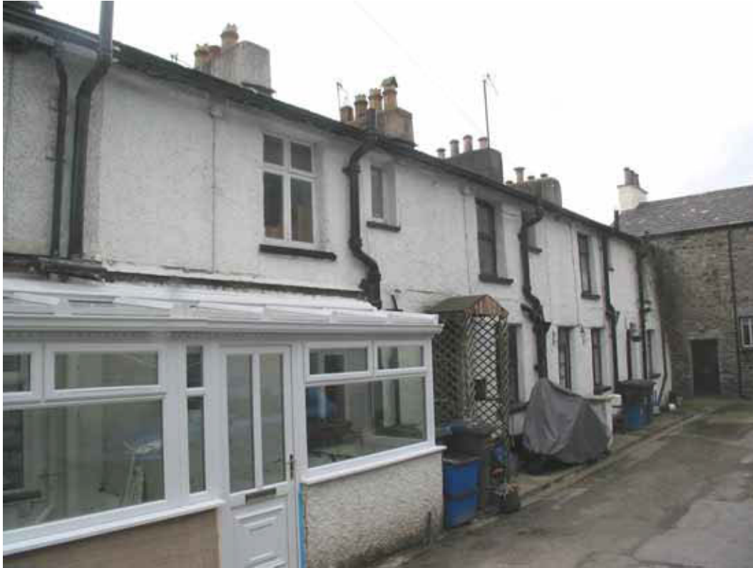
Figure 108: Rear elevations of Nos. 17-20 Low Cottages, Endmoor (Photograph: Simon Taylor 2006, © English Heritage)
