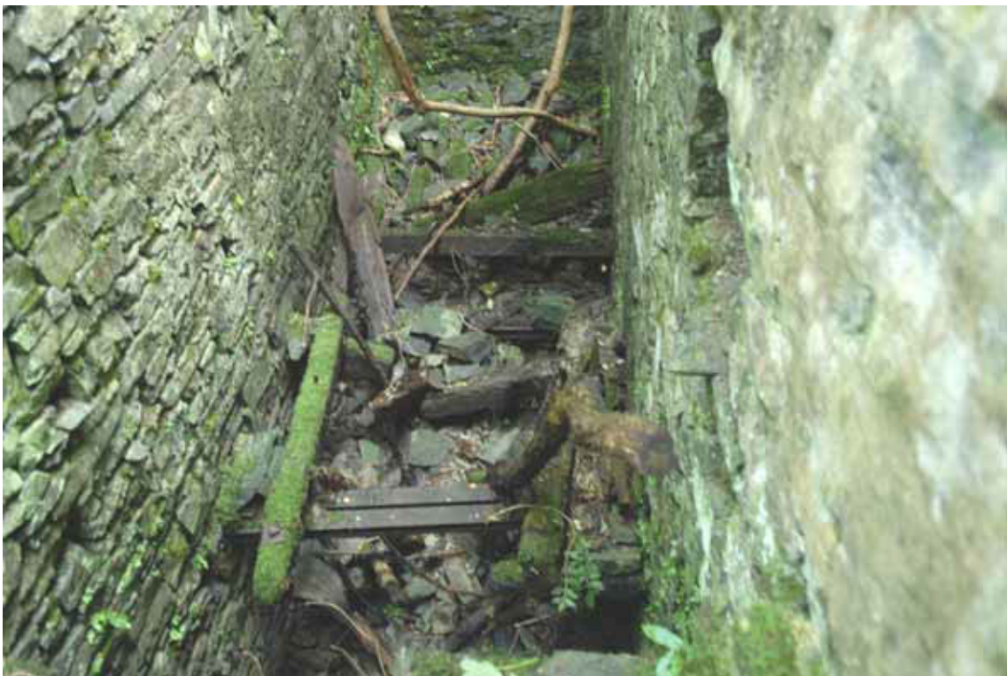
Figure 35: Timber and iron framework to support the base of a flume and turbine in incorporating mill 3 (Photograph: Christopher Dunn 2008, © English Heritage)
