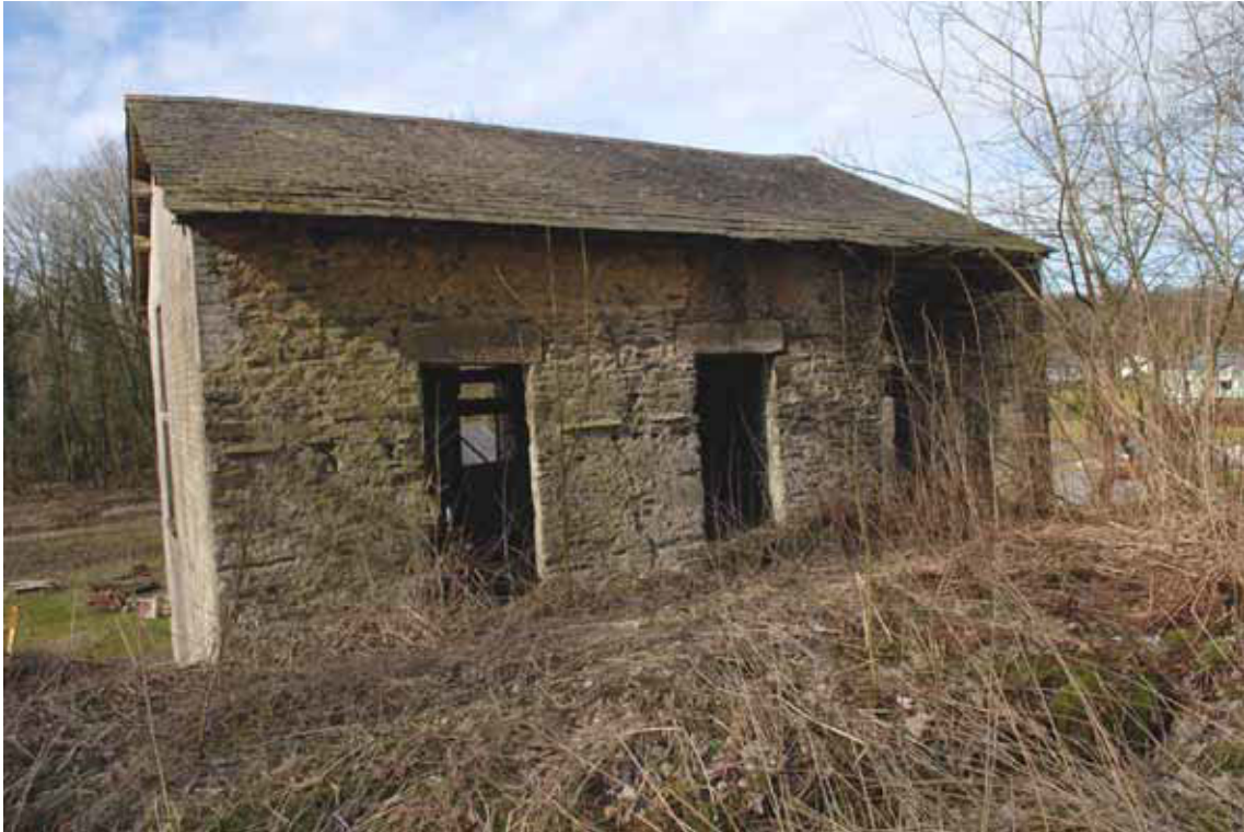
Figure 86: The rear (south) elevation of the sawmill/mechanics' shop (Photograph: Christopher Dunn 2006, © English Heritage)
