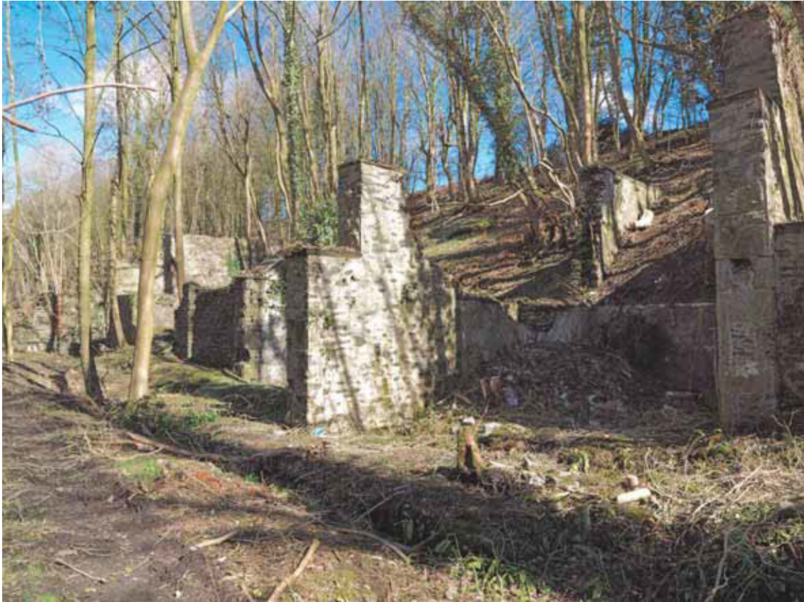
Figure 36: The southern chamber and extended blast wall of incorporating mill 3 (Photograph: Bob Skingle 2006, DP028065 © English Heritage.NMR)
