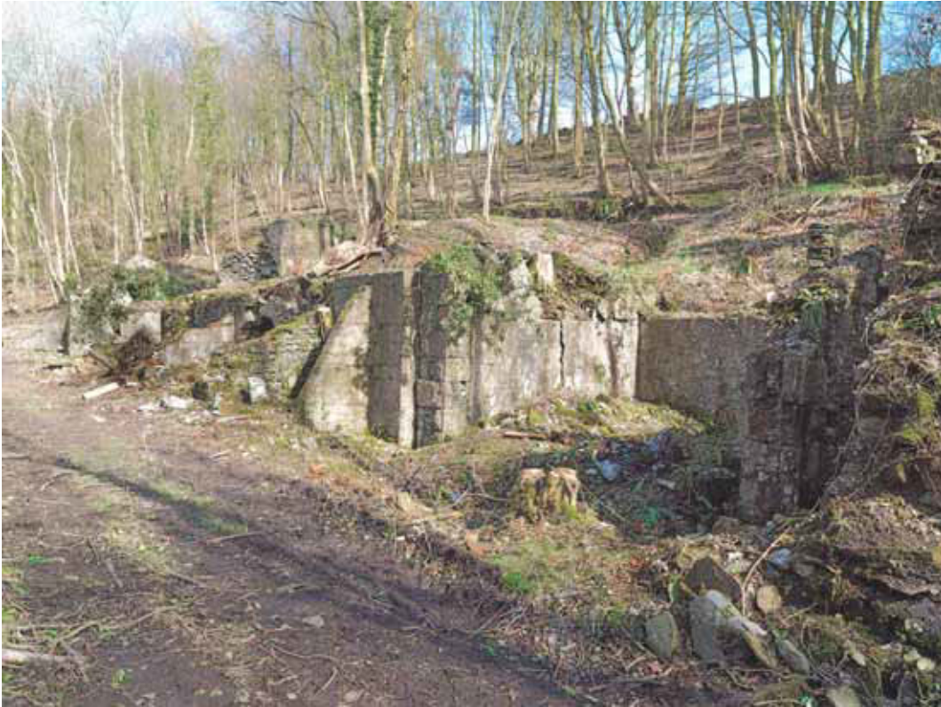
Figure 43: Concrete buttress north of incorporating mill 5 (Photograph: Bob Skingle 2006, DP028074 © English Heritage.NMR)
