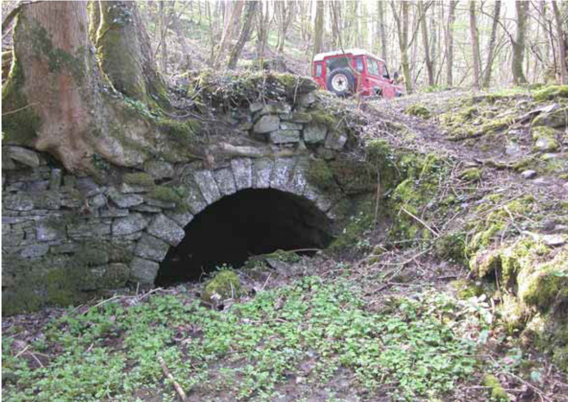
Figure 8: Entrance portal to the high-level culverted leat at the south end of the pre-gunpowder millpond (Photograph: Christopher Dunn 2006, © English Heritage)
