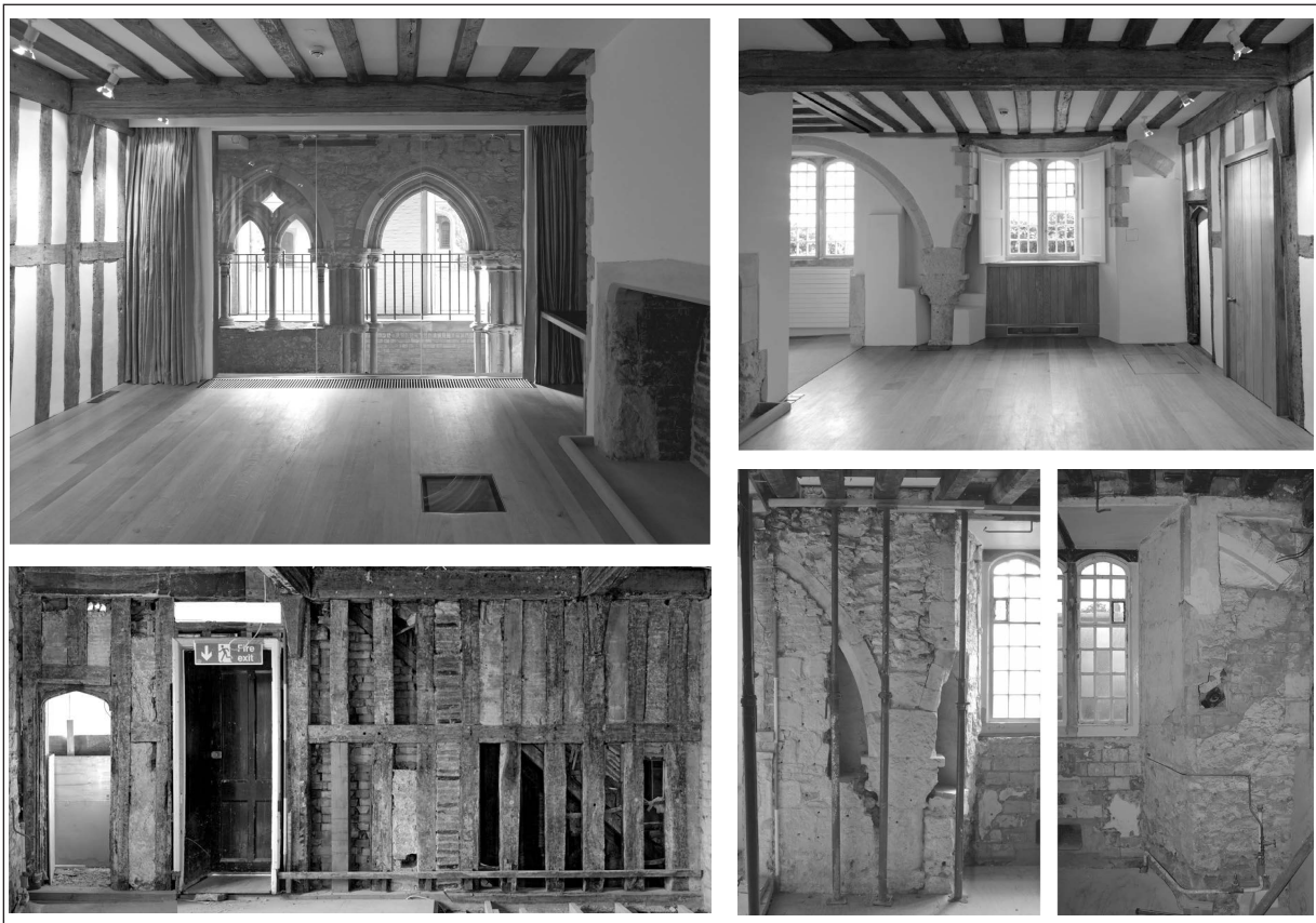
Figure 12. Top, the completed chapterhouse (now meeting room) restoration, facing west (left) and, right, east (note key chapterhouse-component viewing holes in floor; photographs © Tim Soar); below, during renovation works (see Evans et al. 1997 for relevant elevations).
