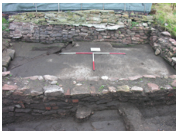
Plate 3. Foundation wall (4/11) of the 'slate shed' showing possible blocked-up entrance at the southern end. From the east.
