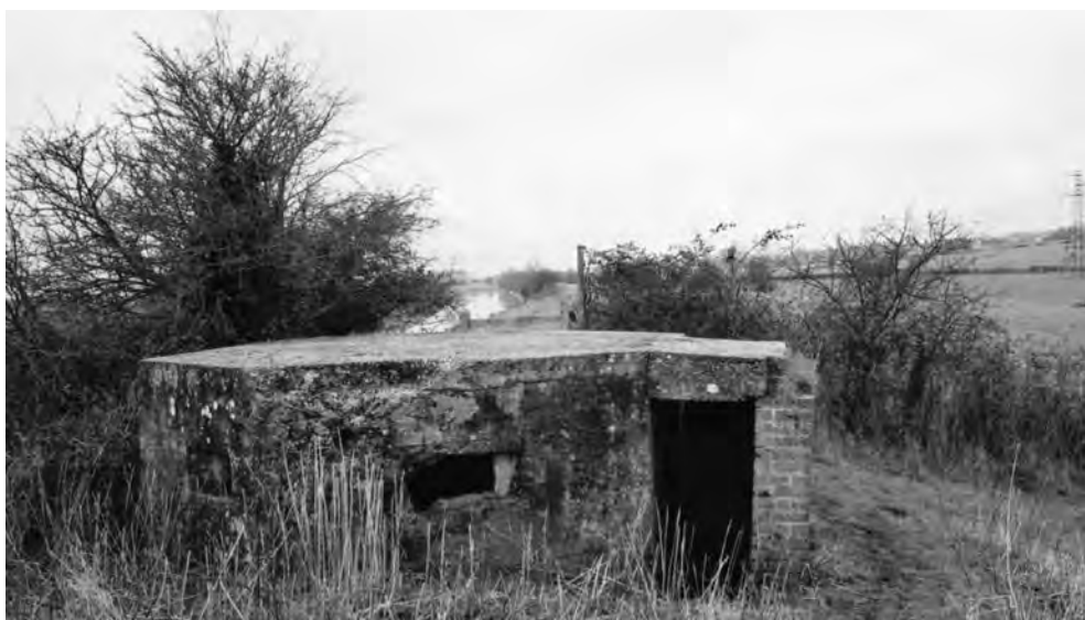
FIGURE 118 Type 22 pillbox [8223] between Bilsington and Ruckinge bridges. Its entry porch is in danger of collapse, and its eastern face has suffered damage at some time. (PHOTO: THE AUTHOR, 12 FEBRUARY 2004)
