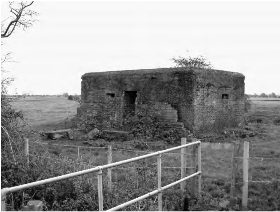
FIGURE 141 Type 24 pillbox [13971]. It has lost a great deal of its exterior brick shuttering and its entry porch has collapsed. (PHOTO: R J C THOMAS, DECEMBER 2004)
