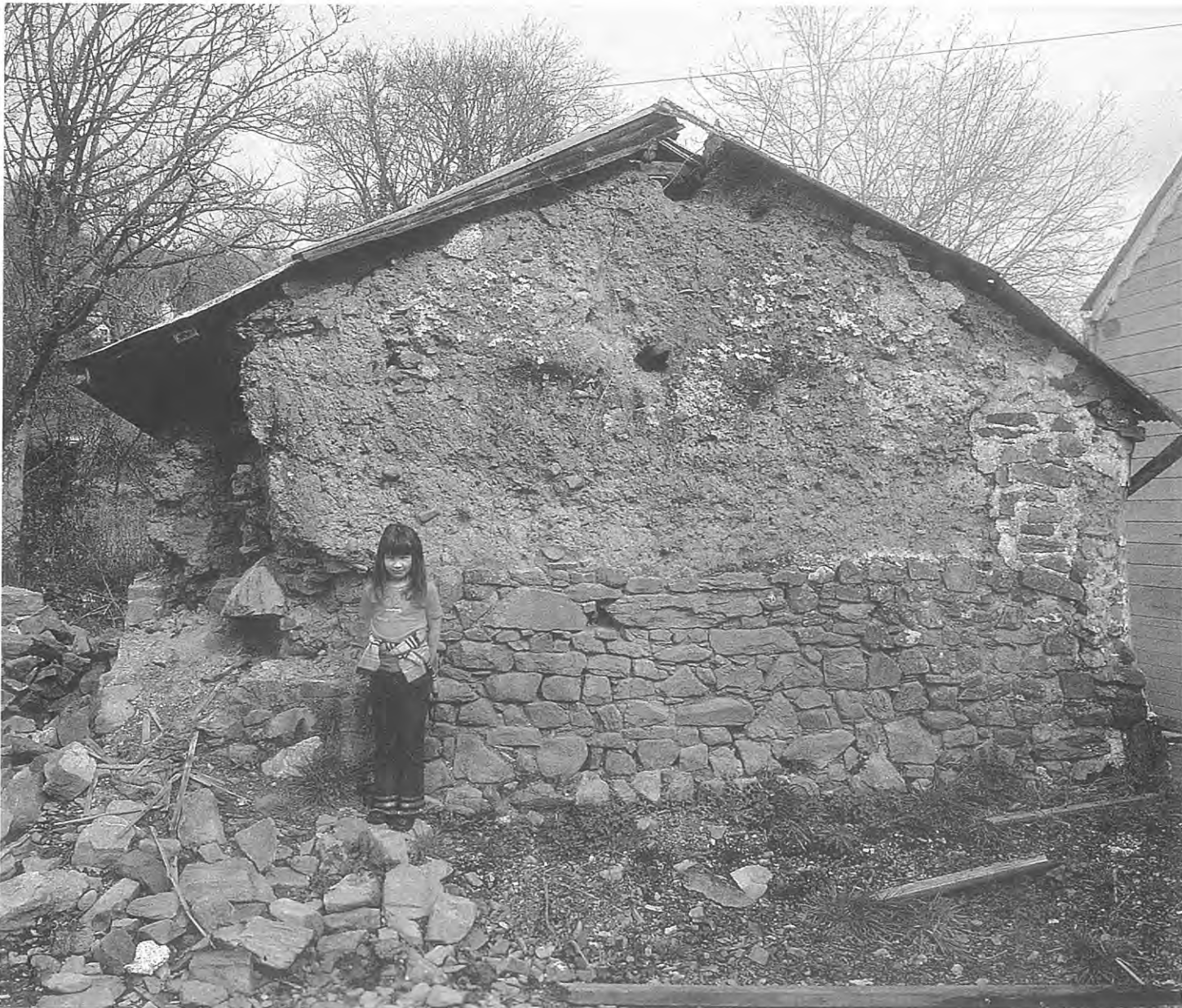
9.4 Clom cottage, Carmarthenshire. An example of an abandoned and rapidly deteriorating clom cottage, once a familiar site throughout rural Wales (photo: Mick Sharp for Cadw)
