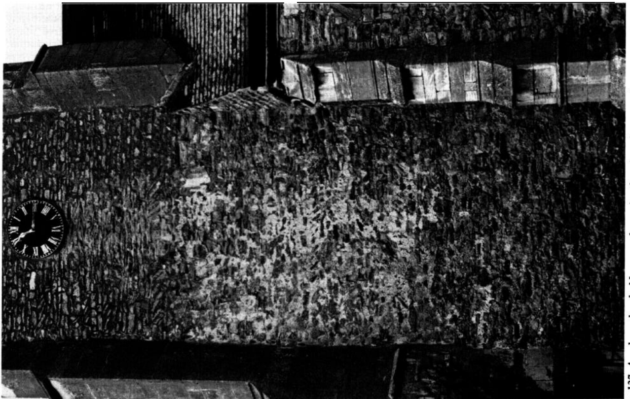
Fig 137 Averham church, Notts: south exterior elevation of tower as it appears to the eye (photo: Christopher J Brooke)
