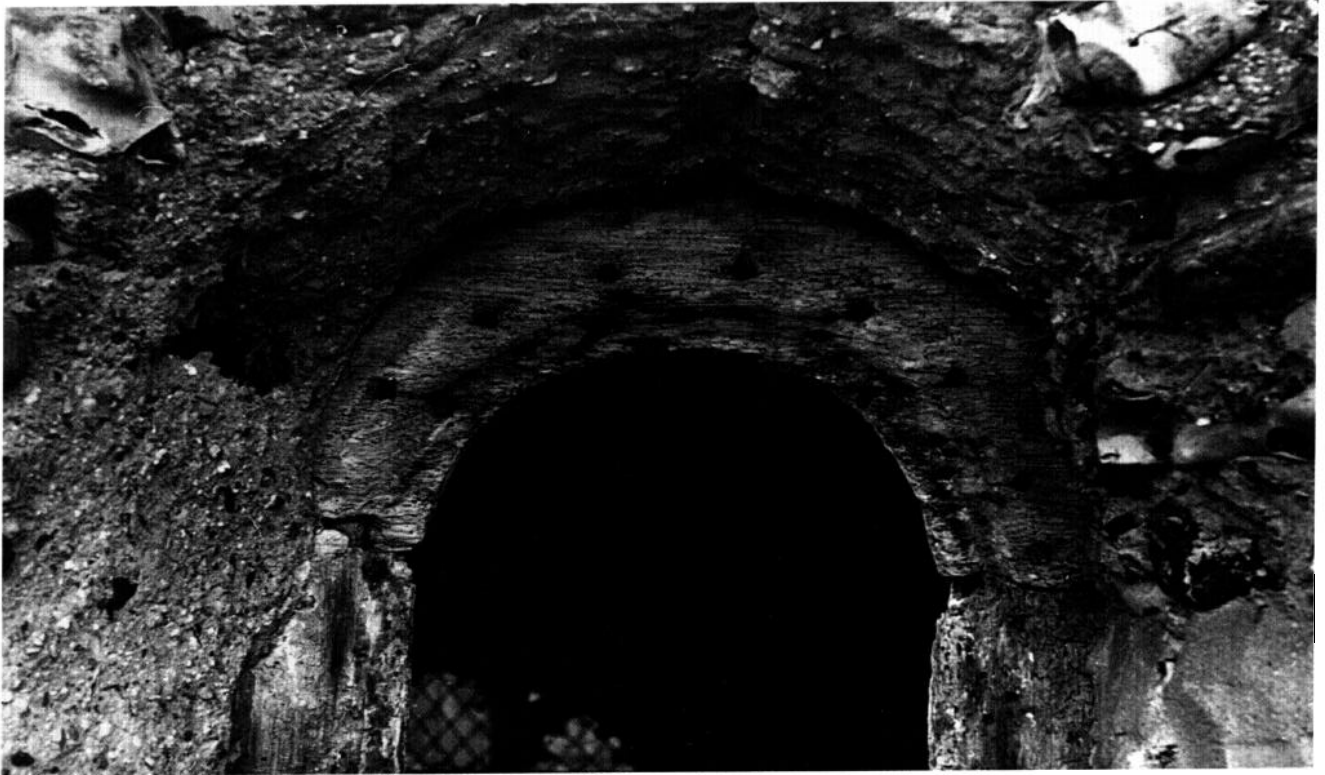
Fig 107 Hadstock: semicircular head of a jointed window frame, showing arc of small holes used to anchor the basketwork hood which served as a forthe arch of flint rubble (photo: W Rodwell)
