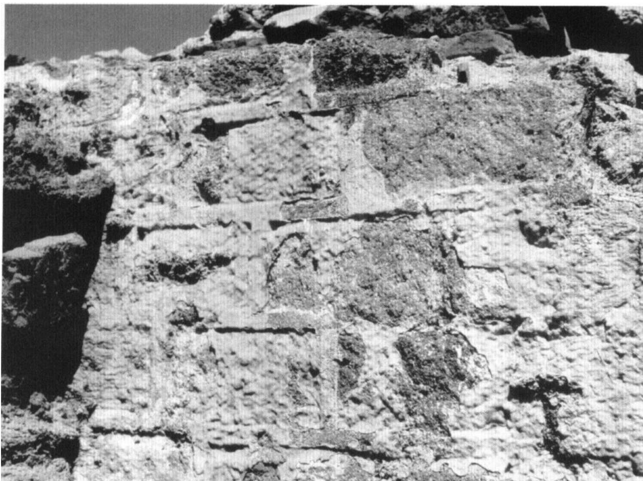
Fig 3.5 Ribbon pointing preserved under a coating of lime scale in the reservoir of the Baths of Caracalla at Ankara. The facing stones are about 150mm in height
