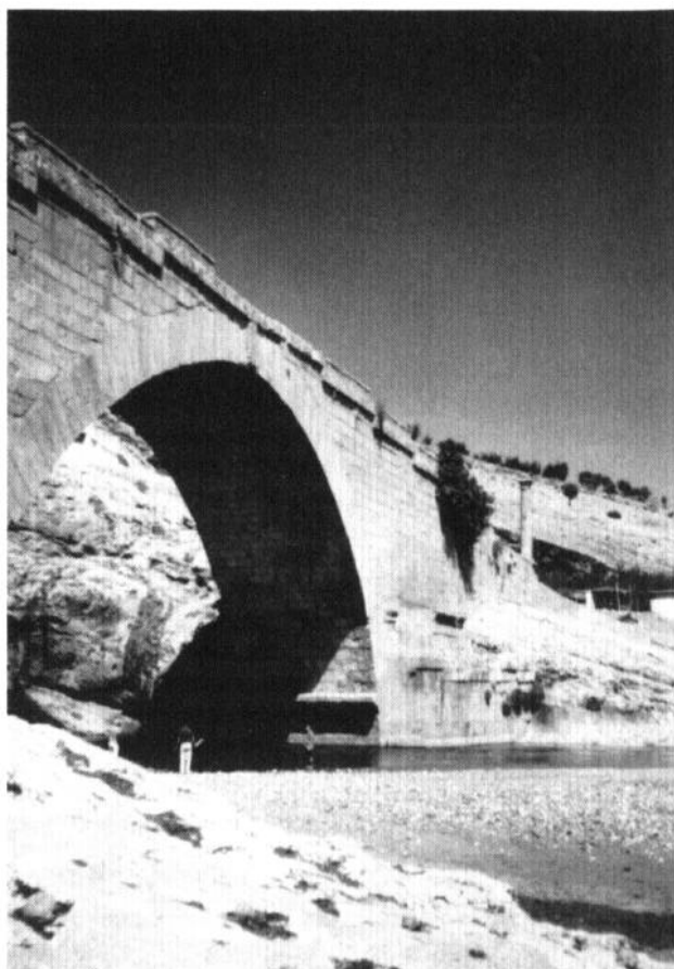
Fig 11.8 The Roman bridge at Cendere (Turkey). Note the column and parapet (N Hodgson)
