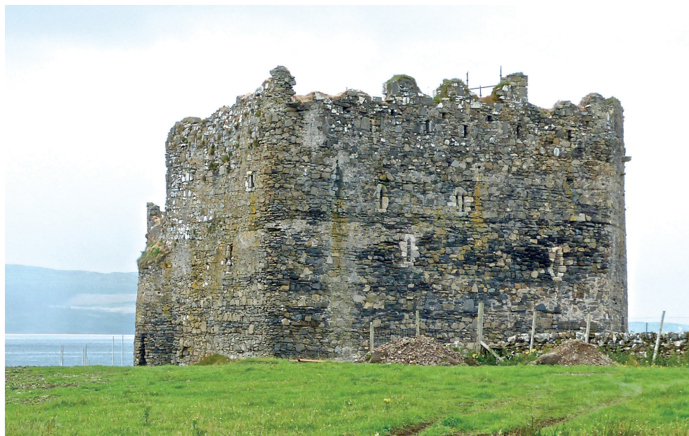
ILLUS 3 The castle from the land showing the blocked-up lancet windows (photo: Jonathon Haylett)
