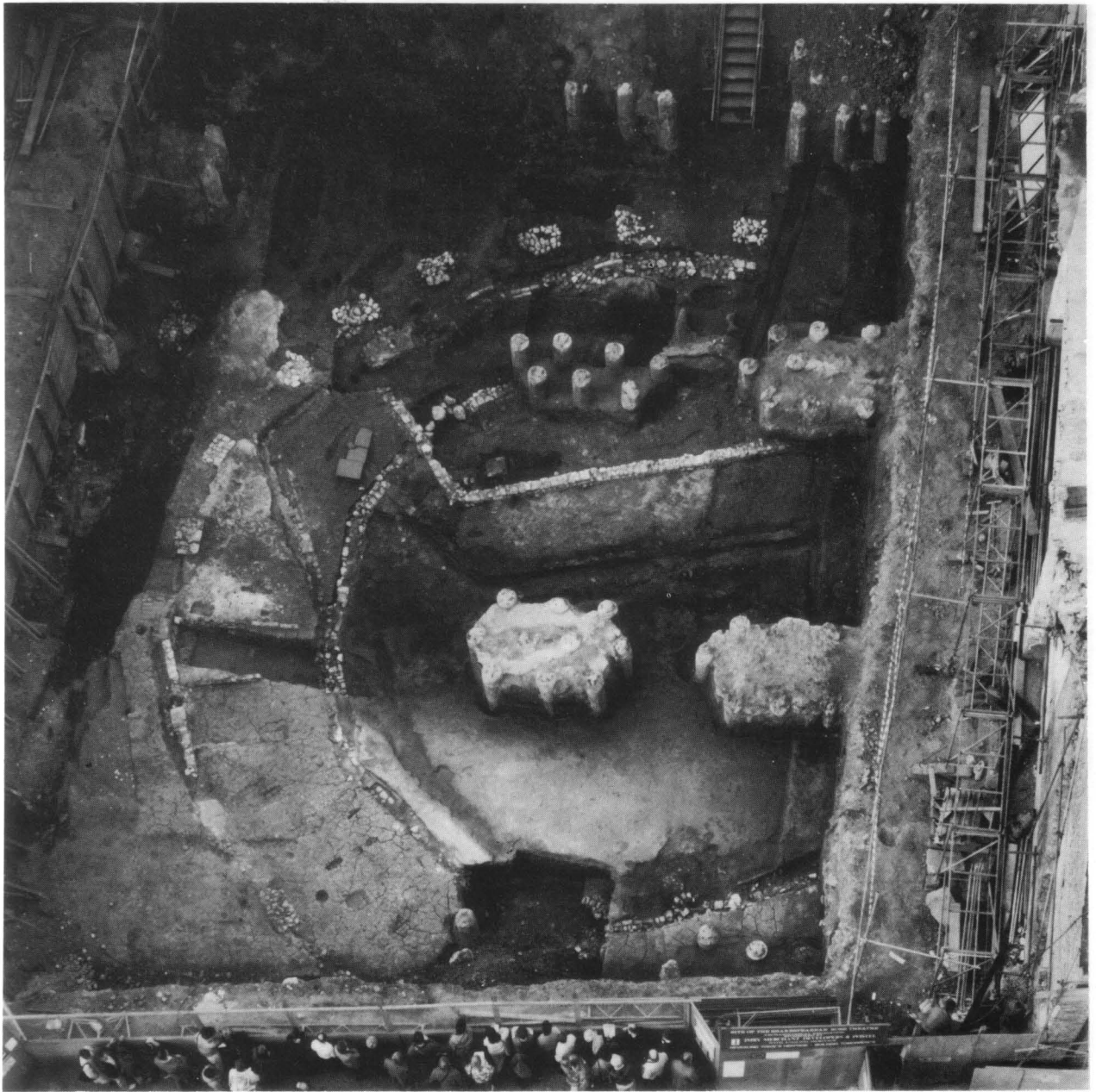
Fig. 4: the Rose Theatre site, from the south. The piles of Southbridge House can clearly be seen in the north and east of the site. Photo: Andrew Fulgoni
