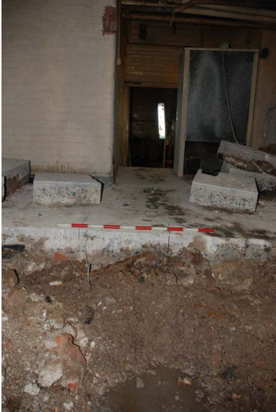
Fig 18 Trench C detail looking east, showing the rubble layer and water ingress below the upper slab. The light in the distance is illuminating Trench A which shows how much higher this part of the site is to the area of Trenches A and B.
