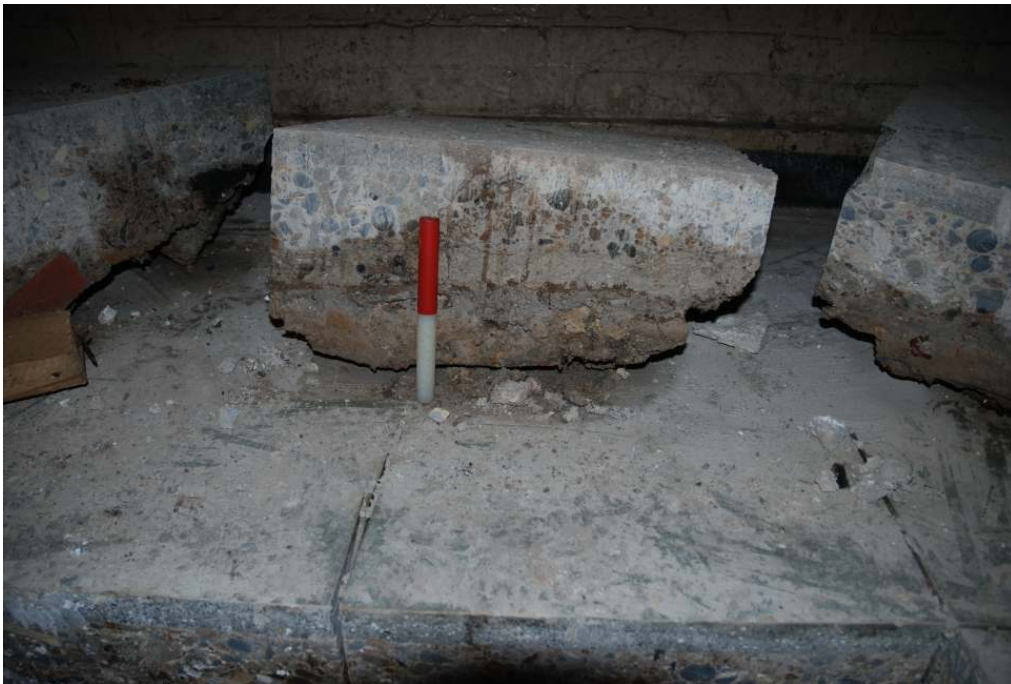
Fig 19 Trial Pit C showing the depth of the upper slab, generally circa 250mm to 300mm depth (Scale 20cm).
