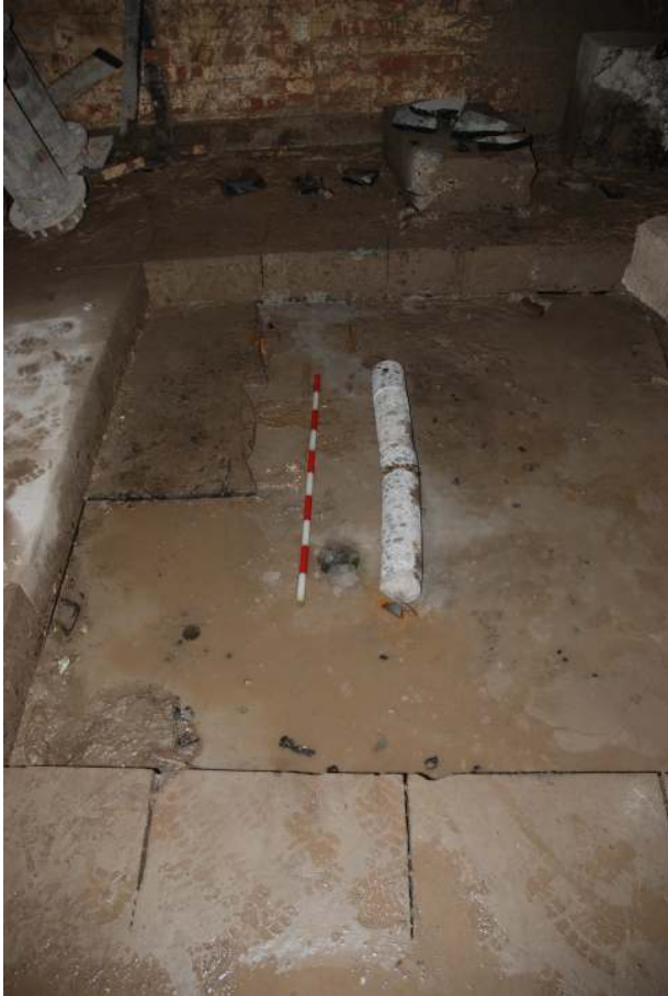
Fig 12 Trial Pit A detail of the concrete bore, which shows the lower concrete slab to be generally 1000mm deep, with circa 200mm of loose poured concrete below this depth. The loose concrete could not be brought to the surface. Adding to this the depth of the upper concrete slab of c 300mm, the total depth of the two concrete slabs and the loose poured concrete beneath the lower slab in Trench A was c 1.5m. The height of the upper slab i.e. the existing basement floor at this point is +0.832m OD, this gives a reduced level for the underside of the concrete to be -0.668mOD.
