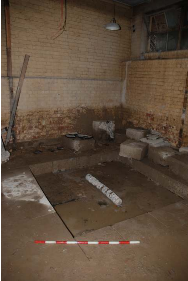
Fig 10 Trench A after removal of the upper basement slab by mechanical saw and after removal of the core of the lower slab, looking east towards the rear wall of the Nurses' Accommodation building (Scale 1m). The upper slab has been cut through in an area 2m 2 , top of basement floor at +0.832m OD
