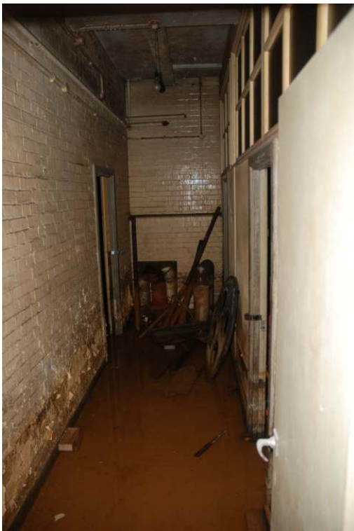
Fig 9 General location of Trench A at the rear of the basement on the southern side, prior to the removal of the partition wall on the right of the image.
