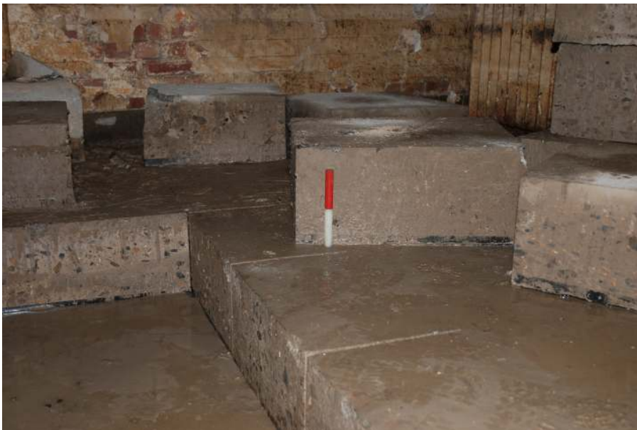
Fig 11 Trench A showing the depth of the upper slab, generally circa 250mm to 300mm depth (Scale 20cm).
