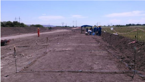
Photo 1. General view of the excavation site following topsoil stripping. View to east.
