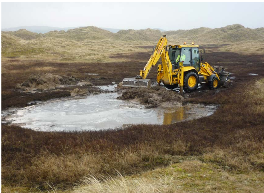
Plate 5: Typical observation during the excavation of a toad scrape in dune area
