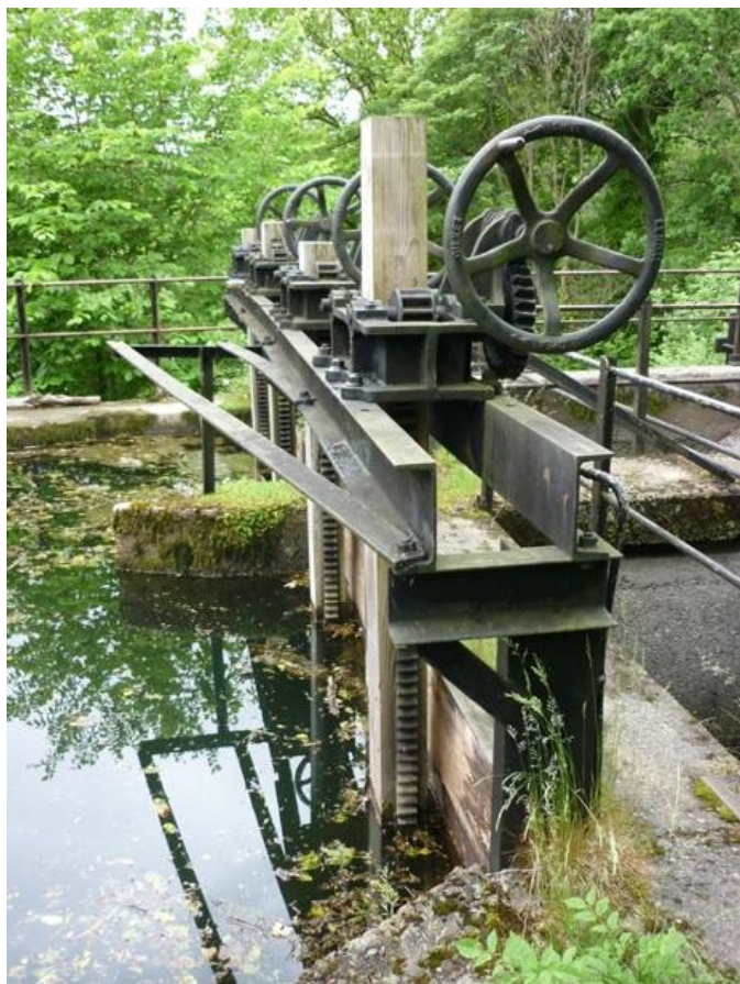
Plate 5 (left): Sluice gates at the power house
