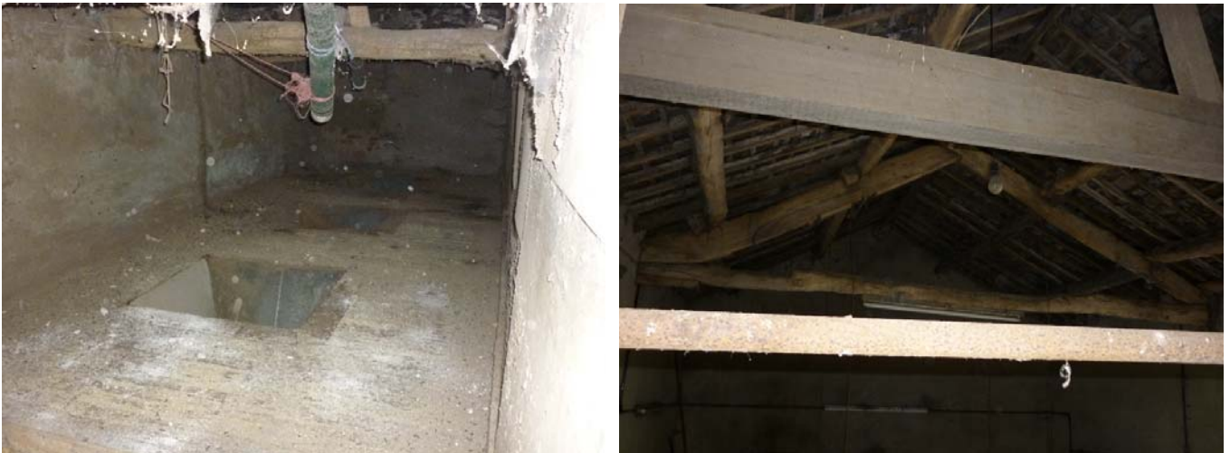
Plate 37 (left): Feeding chutes in the floor above the west end of Building 3
