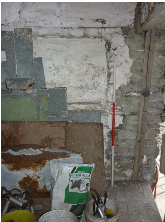
Plate 30: Blocked aperture to the south side of the east elevation on the upper floor of Building 2
