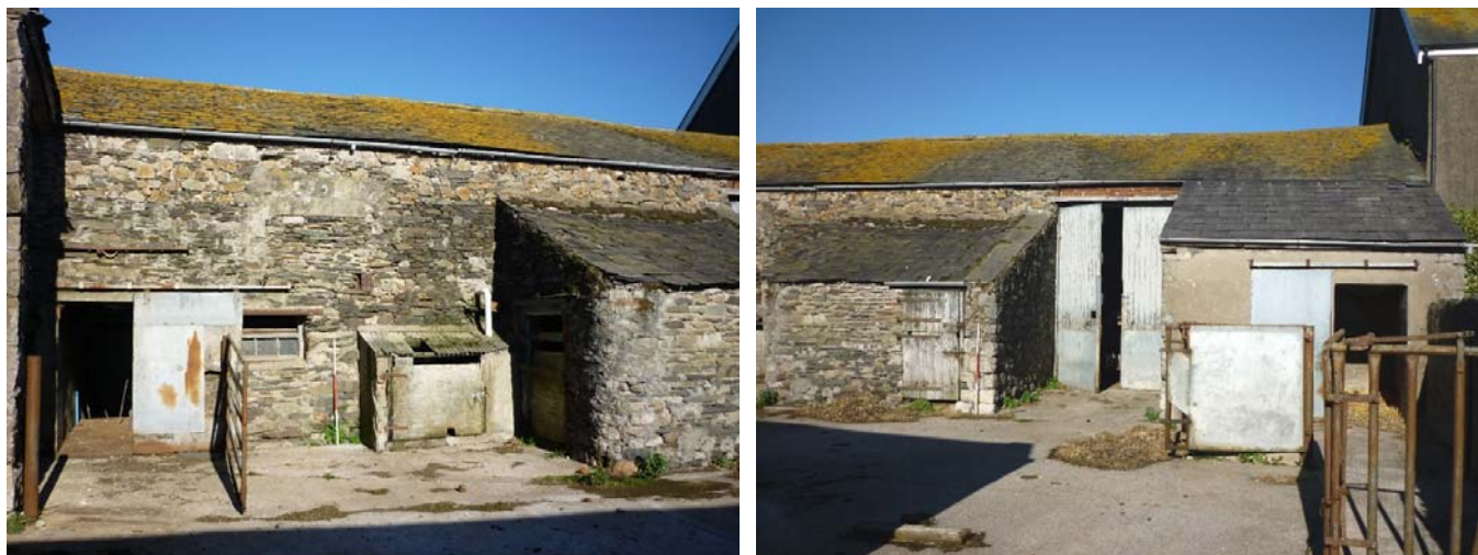
Plate 20 (left): West end of the south elevation of Building 3 and Building 3a
