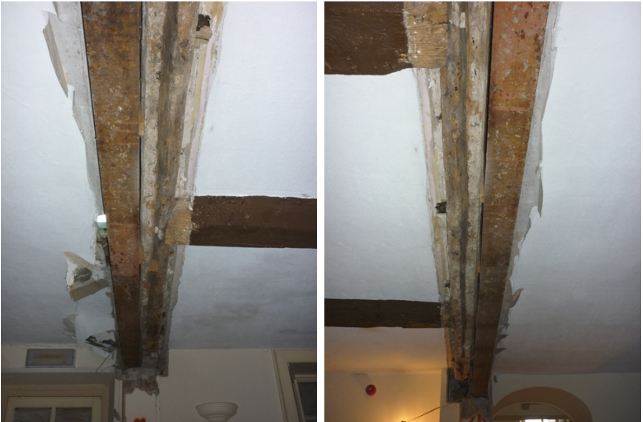
Plate 19 (left): East end of the iron and timber beams in Room G10
