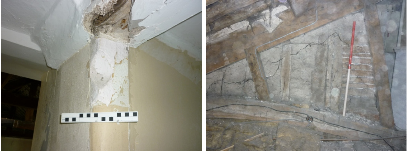
Plate 41 (left): Moulding on the west edge of the chimneybreast on the north side of Room F9
