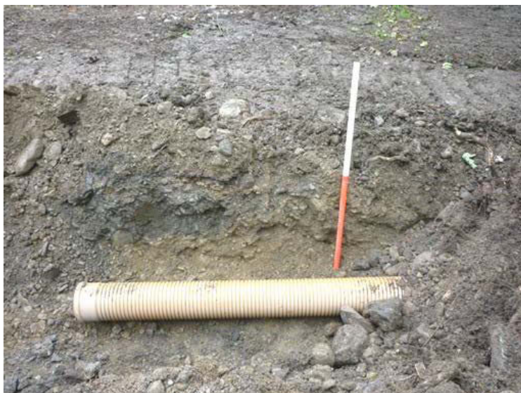
Plate 14: Possible original ground surface (04) and slag deposit (05) at the west end of the service trench
