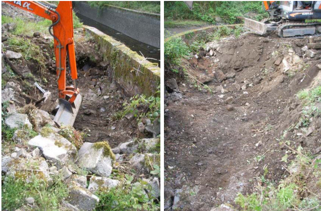
Plate 3 (left): Overburden being removed by machine from the north-east end of the excavation area
