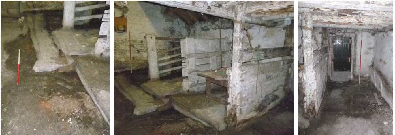
Plate 51 (left): Uneven concrete floor and drain in Ground Floor Room 7
