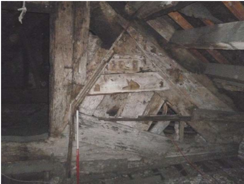
Plate 67: Panelling and attached newspaper cuttings, north face of north truss, Room A2
