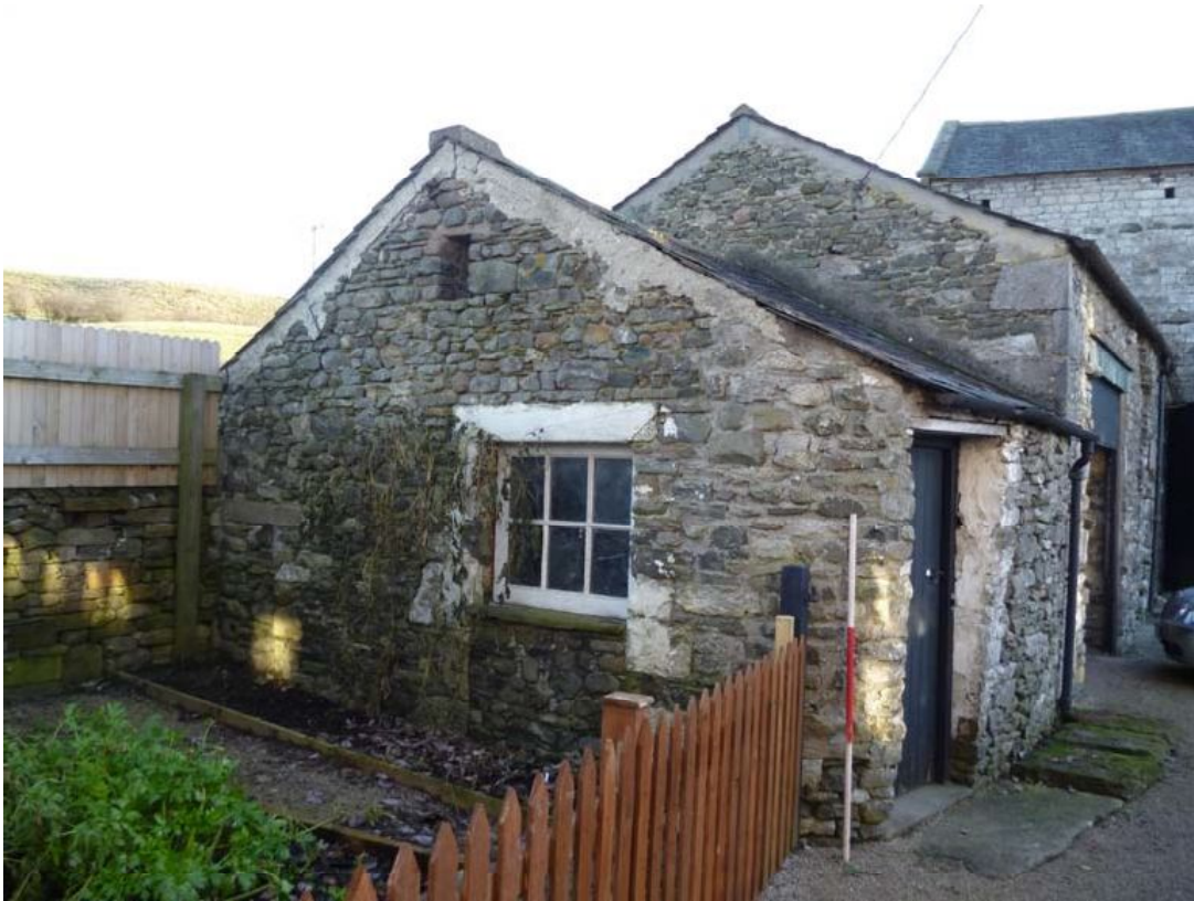
Plate 8: North end of the outshut to the north, comprising the north-east end of the north-west external elevation
