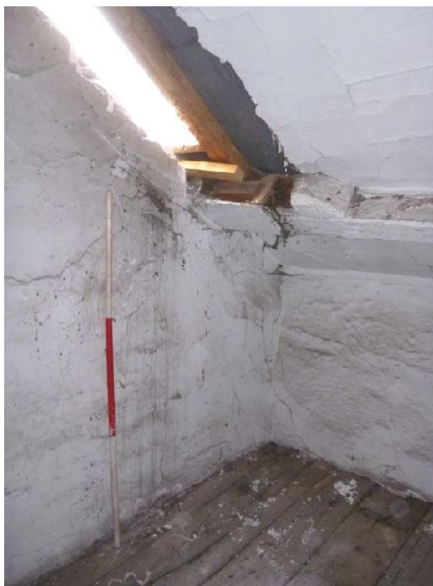
Plate 166: Modern skylight and block attached to purlin, north-west side of Room A3
