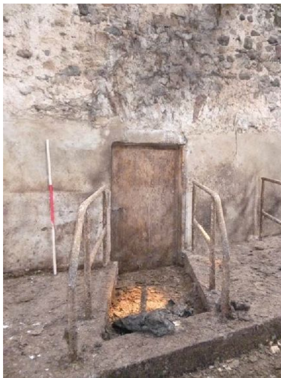
Plate 113: Doorway in the south-east elevation of Room 2, Building 5, set within an earlier voussoir arch
