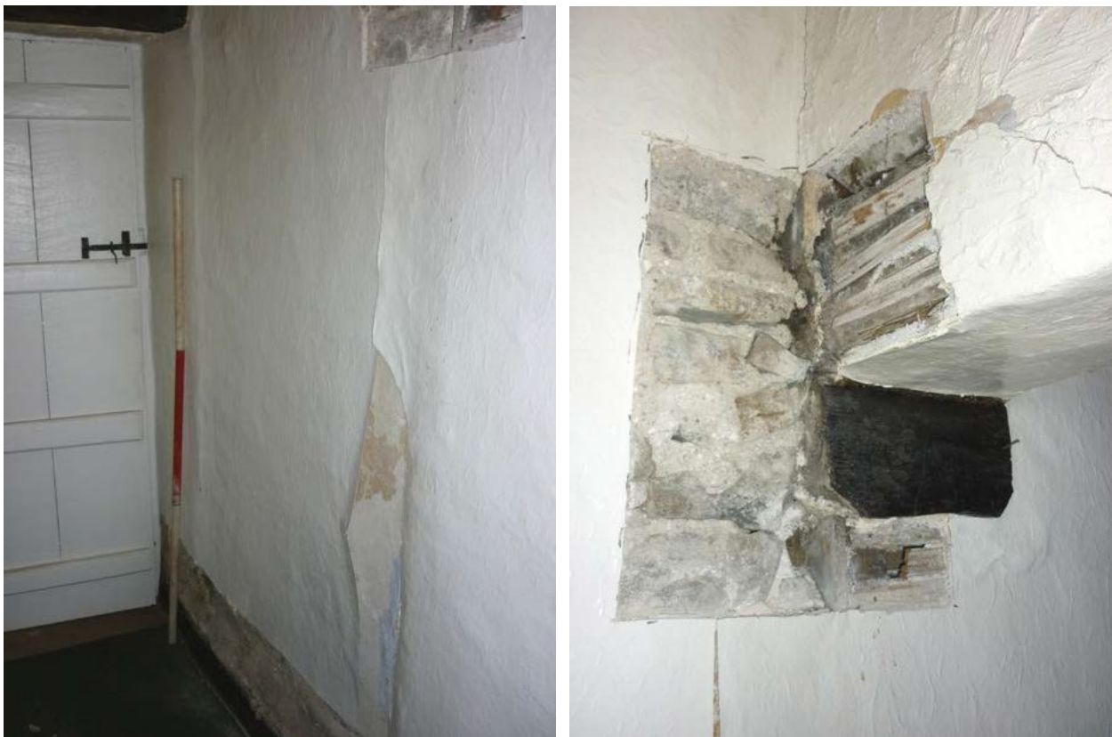
Plate 6 (left): Blocked area on east side of Room G8
