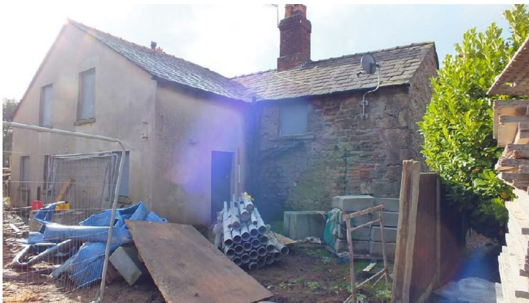
Plate 7: The north-west end of the north-east external elevation, viewed from the north
