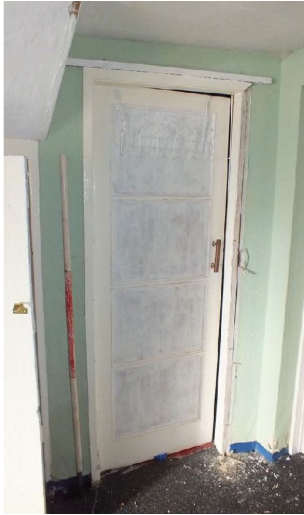
Plate 31: Door at the north-east end of the north-west elevation, Room G4, viewed from the south
