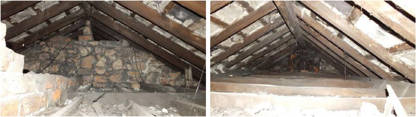
Plate 84 (left): General view of the roof space above Room F6, viewed from the south-west
