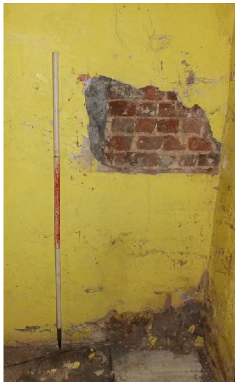
Plate 47: The junction at the north-east end of the north-west elevation, Room G8, viewed from the south-east
