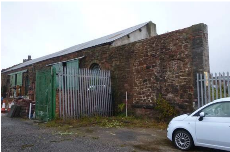
Plate 25: Truncated wall finished with concrete block at the east end of the south external elevation
