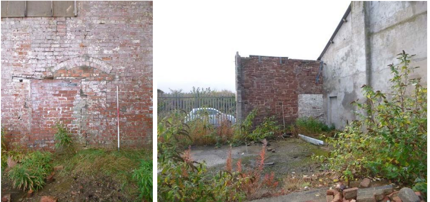
Plate 18 (left): Blocked doorways in the east end of the north external elevation
