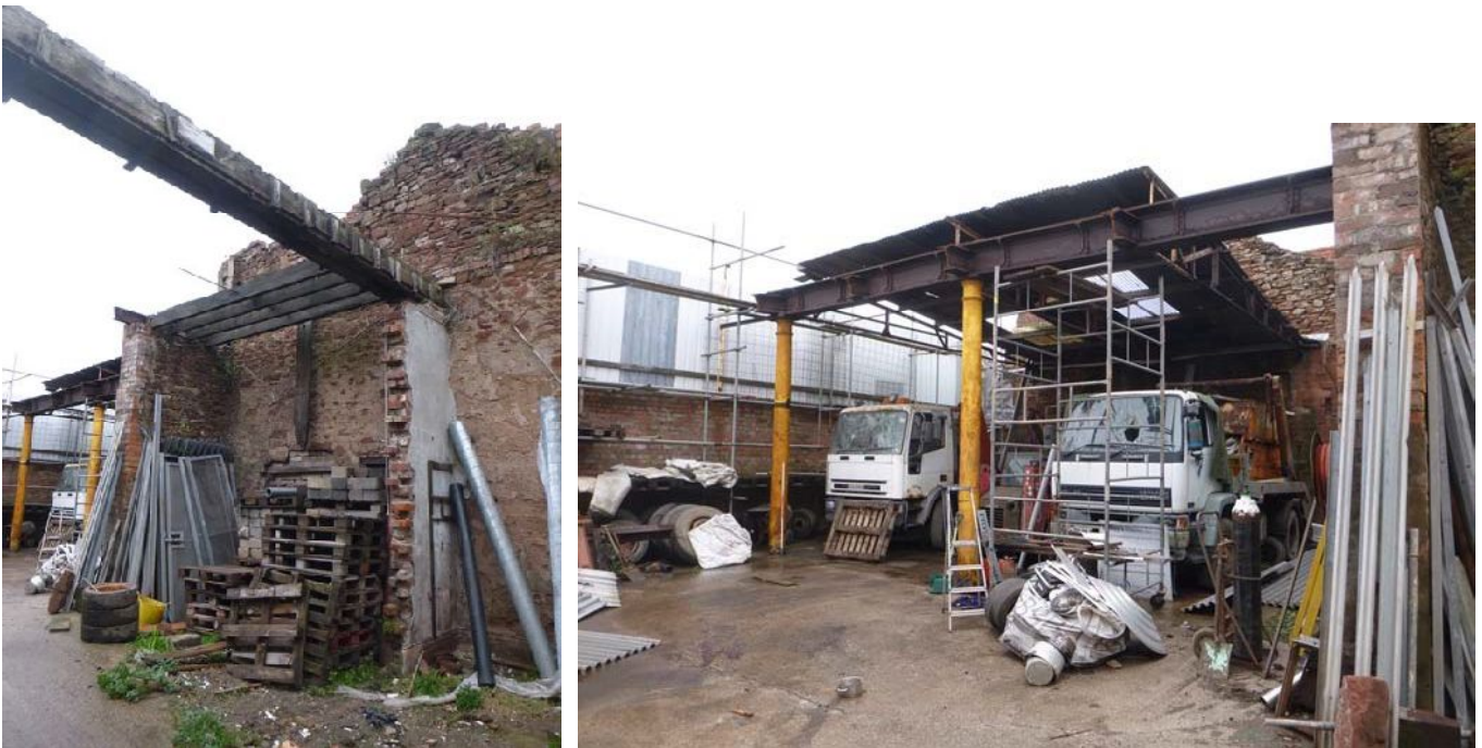
Plate 32 (left): Large east/west beam and joists on the south side of Room G1
