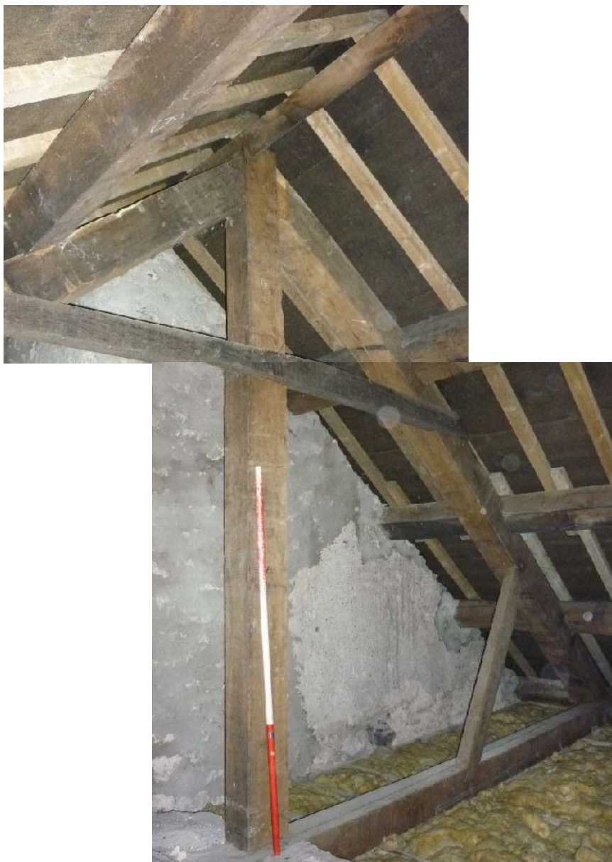
Plate 69: Composite photograph of the truss in the roof space to the east of Third Floor Room 2
