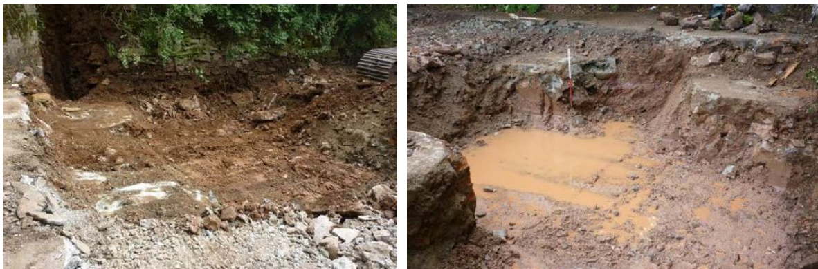
Plate 7 (left): Concrete stanchions (to the left) and retaining wall (to the rear)
