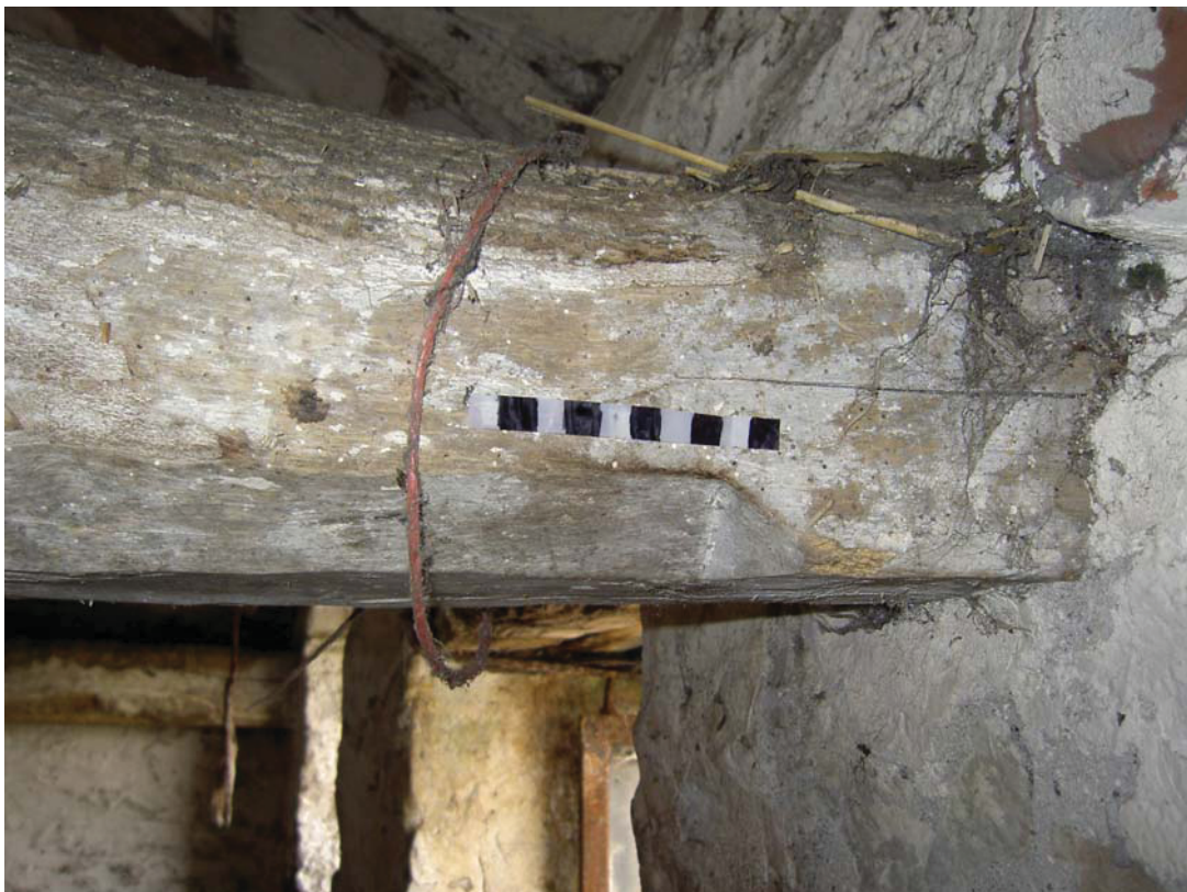
Plate 19: Detail of stop-chamfer decoration at south-east end of tie beam in ground floor Room 4
