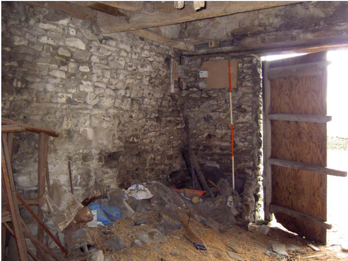
Plate 17: Lower ground floor Room 3, wagon doorway in south-west side and alcove to south-east (following clearance)
