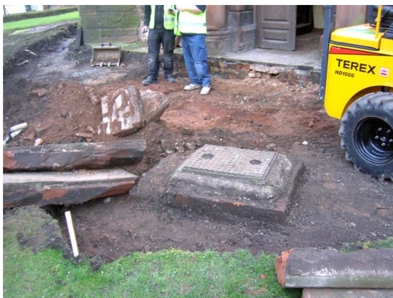
Plate 8: Area 3, outside tower at west entrance of church, showing modern drain cover
