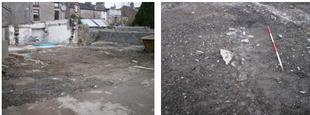
Plate 8: (left) Site following the removal of the concrete surface ( 100 ) showing the concrete block walls
