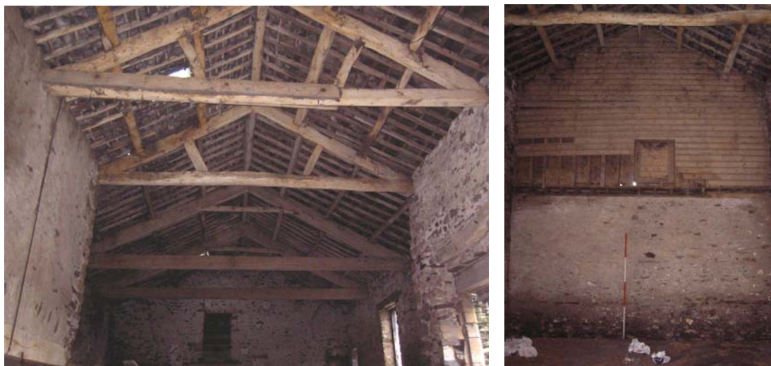
Plate 25: Trusses in the south threshing barn and above the south central shippon
