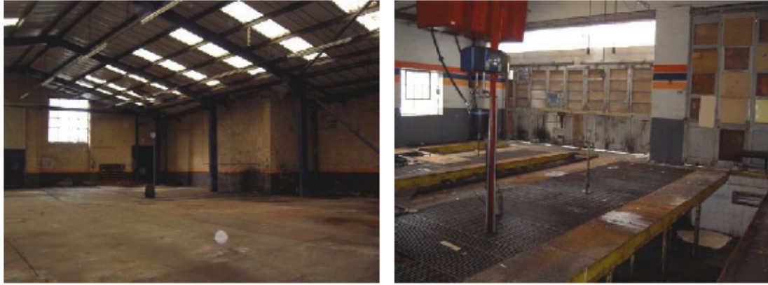
Plate 6: (left) Interior of the western garage buildings showing steel frame structure and concrete floor
